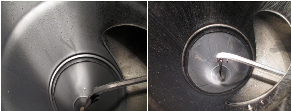
Typical flue interior after testing without the Oeko Tube in operation during the test
