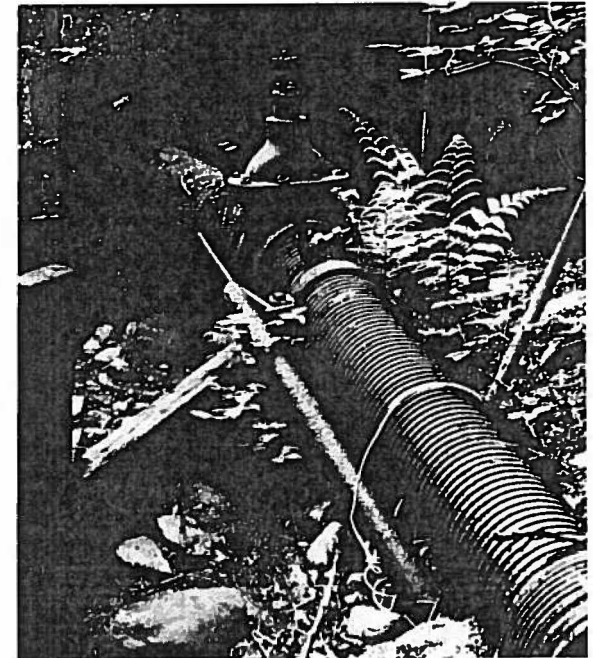
Boom is stretched across a creek to stop oil from a pipeline spill.
