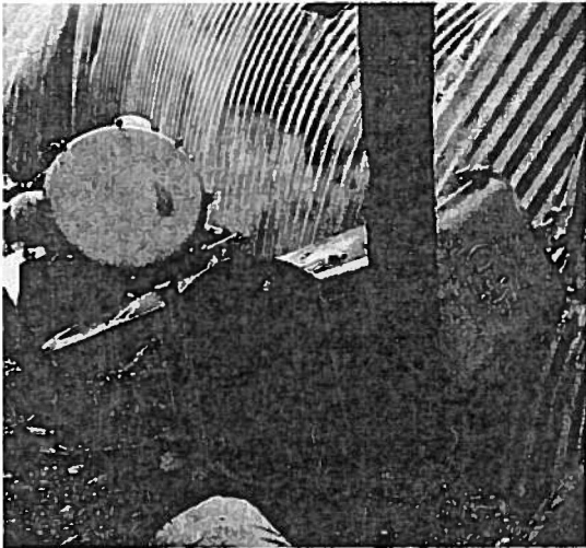
Old electrical transfonners, like these three at an abandoned military site, can contain hazardous wastes, such as PCB's.
