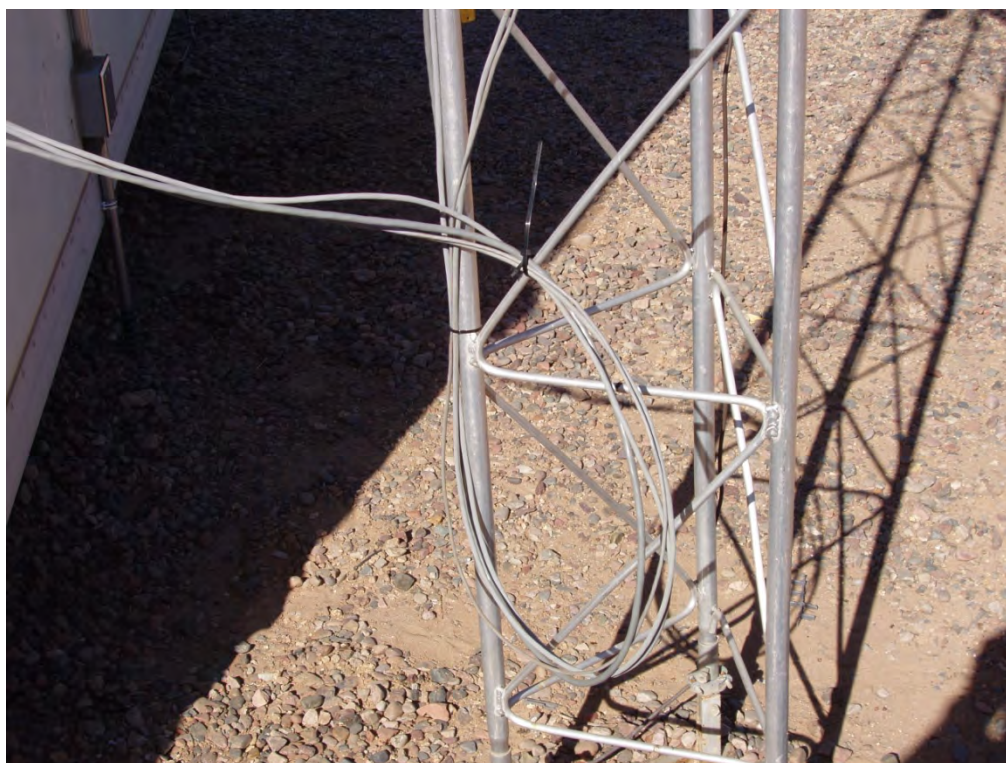
Figure 1.13 Signal Cable at Tower Base
