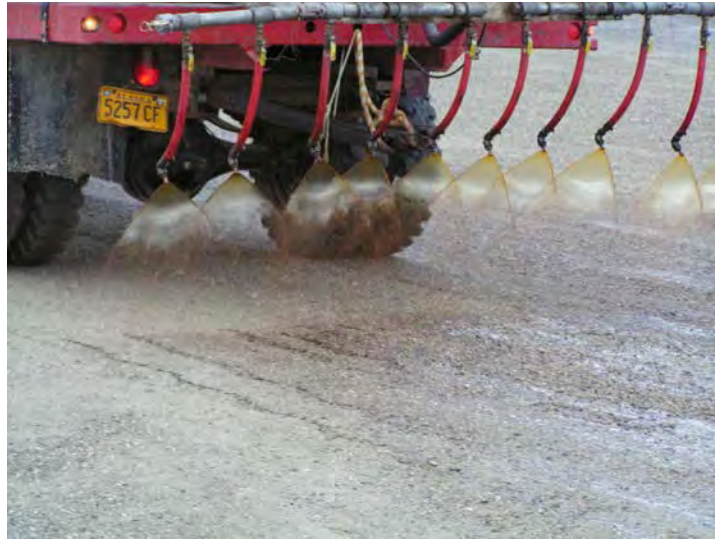
Figure 5.11 Uneven fan distribution
