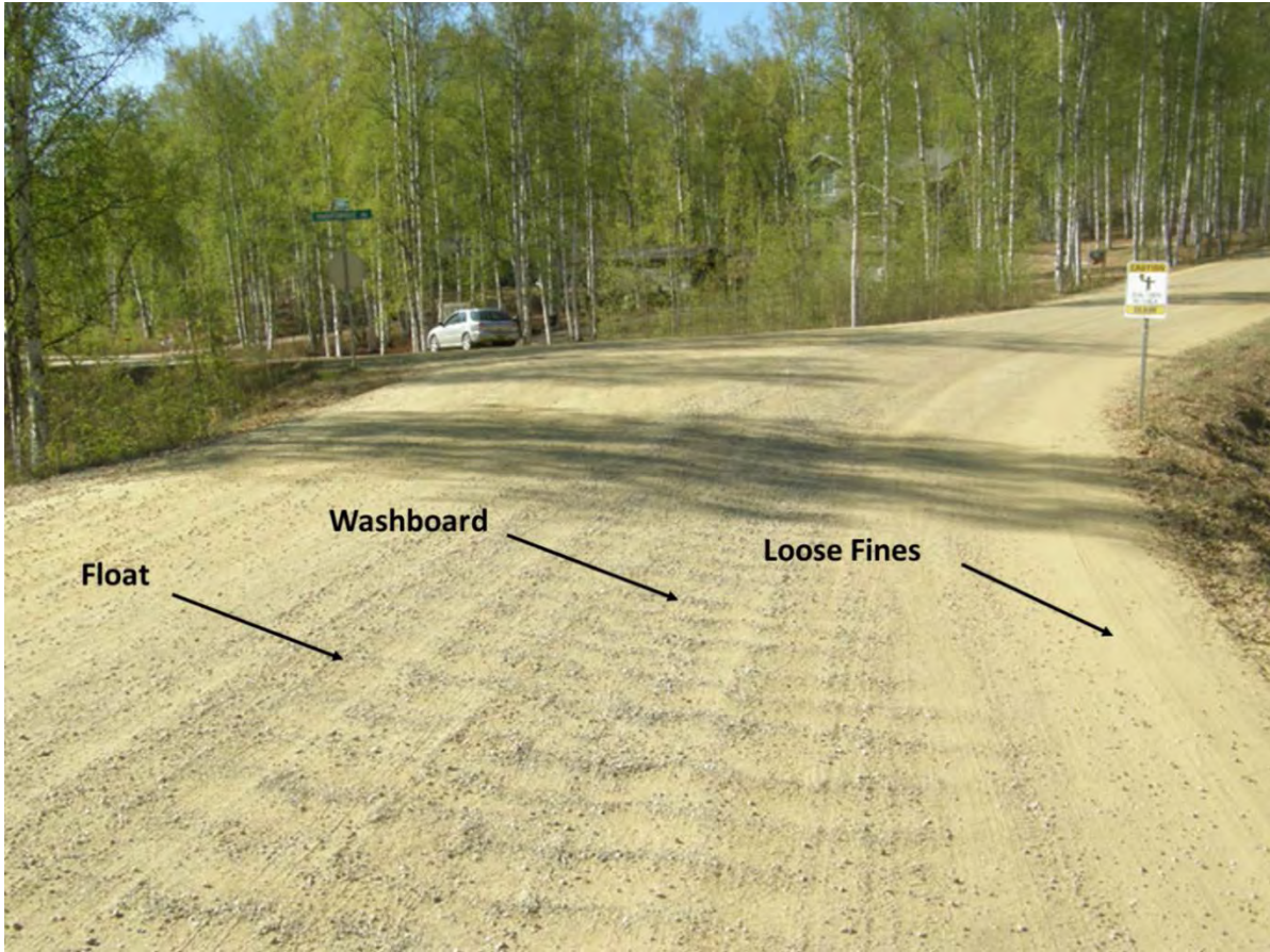
Figure 4.3 Attributes of gravel road distress
