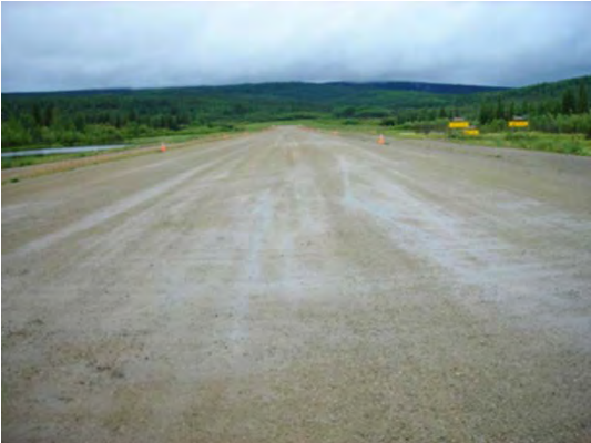
Figure 4.6 Proper crown after rain
