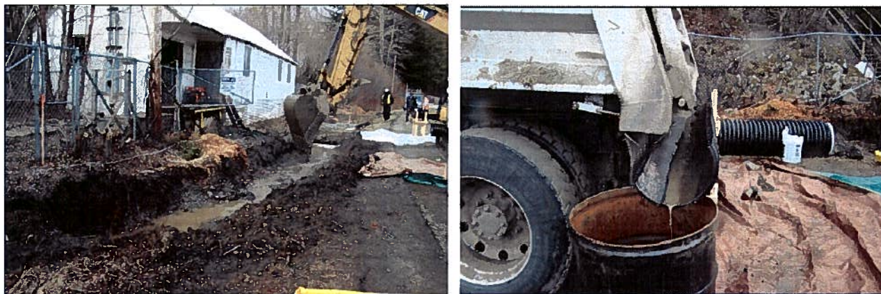
Figure 6. Front Street ditch at the warehouse; draining water from the contaminated soil into containers.
