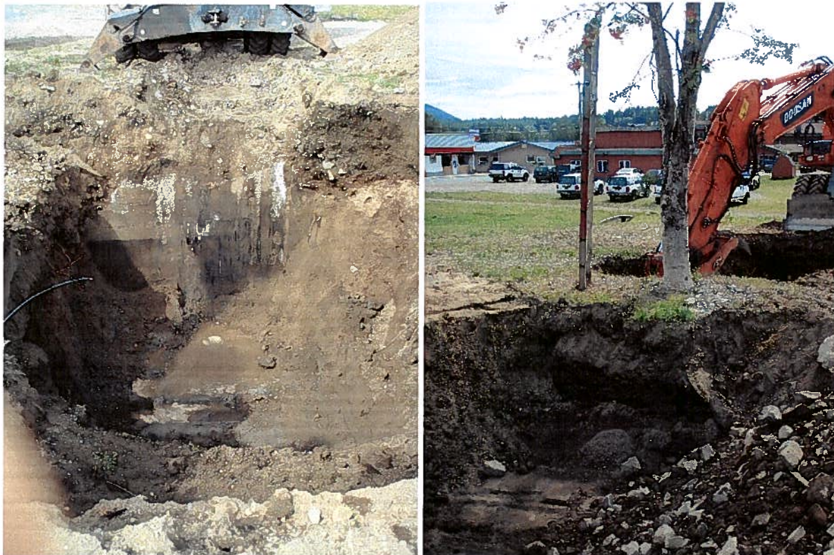
First excavation: looking west at the foundation wall and south at the tree hindering excavation.
