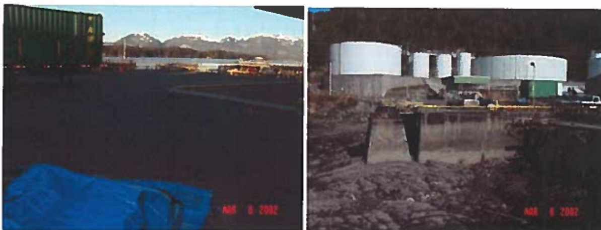
Figure 4. 2002 Site Assessment photos show the excavation site and its distance from the bulkhead.
