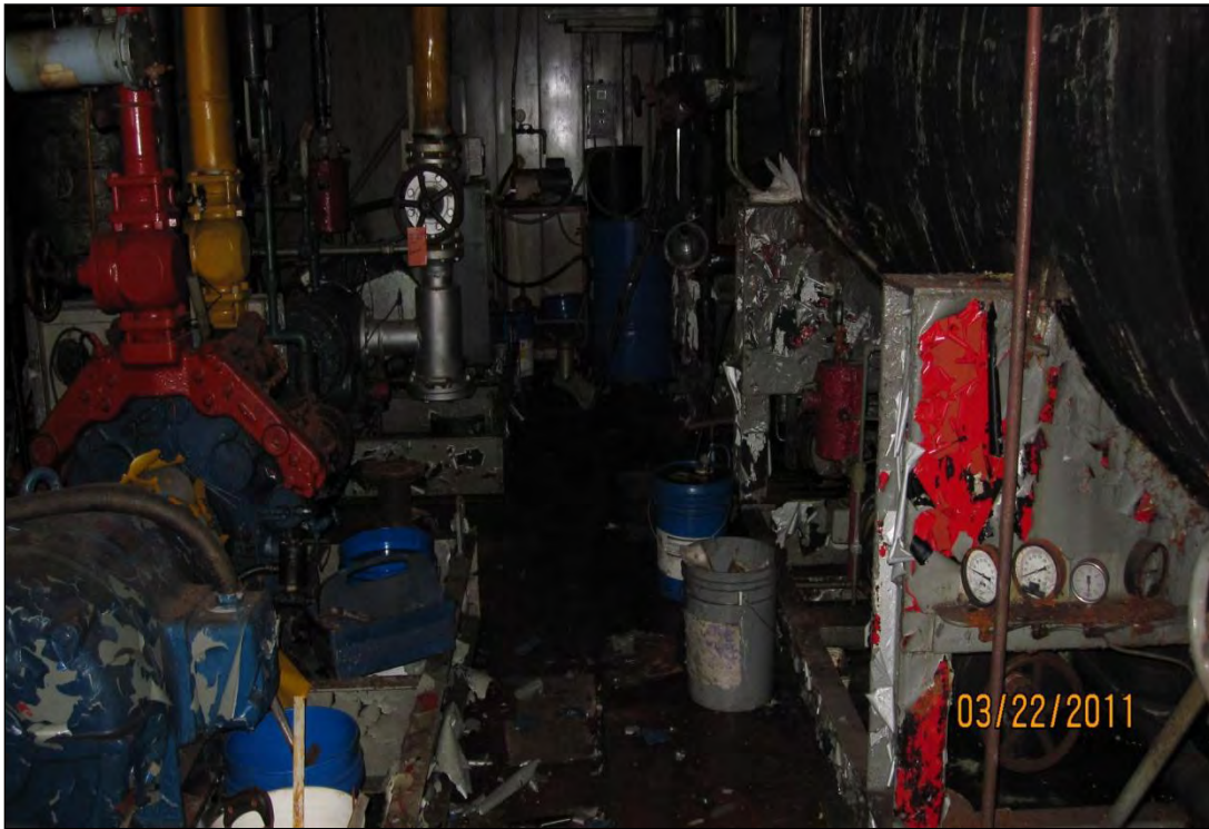
Photo 6. Blistering and peeling paint located inside engine room building.
