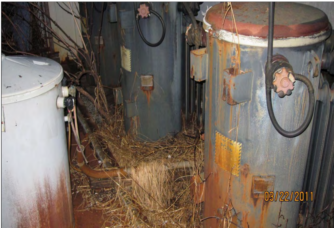
Photo 23. PCB bearing transformers located on the west exterior wall of the engine room building.
