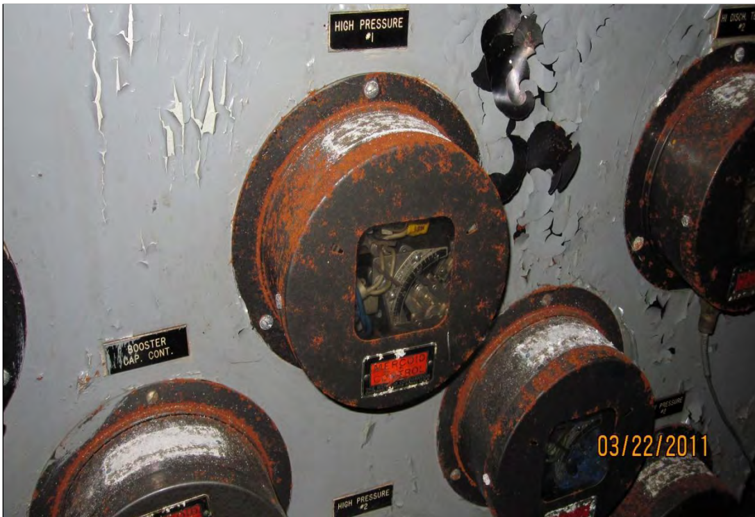
Photo 4. One of several banks of mercury switches for the ammonia refrigeration system in engine room building.
