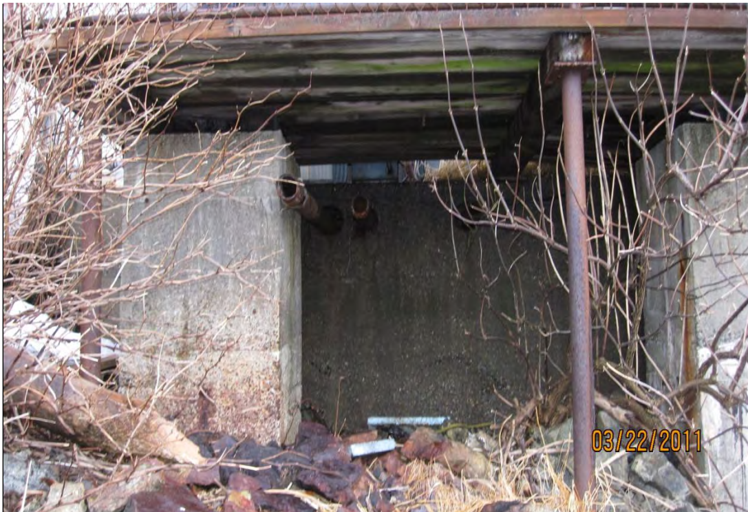
Photo 25. Open pipes protruding from west foundation wall of engine room building.
