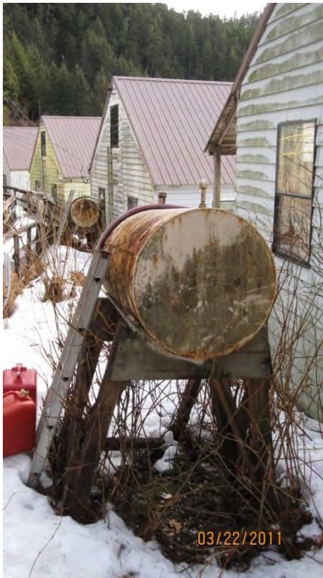
Photo 19. Company housing exterior heating oil ASTs.
