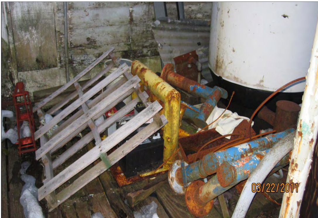
Photo 3. Batteries located on exterior east side of engine room building.
