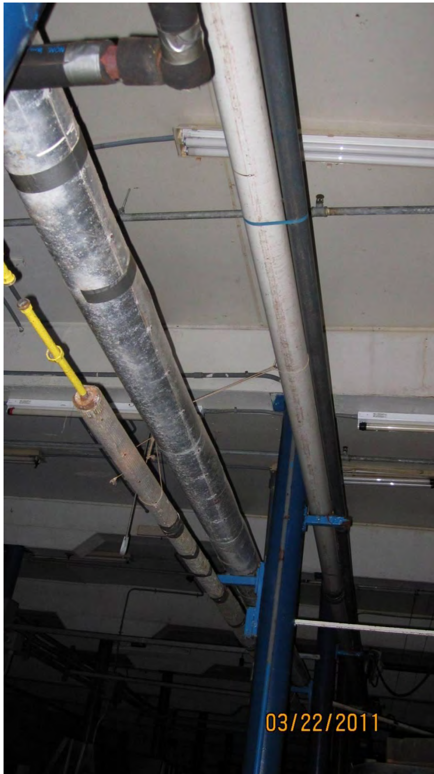
Photo 5. Potential ACM pipe insulation located on yellow pipe in photograph. Pipe is located inside crab plant building.
