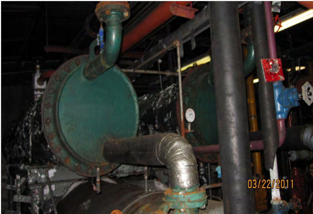
Photo 7. Refrigeration system receiver tank inside engine room building.
