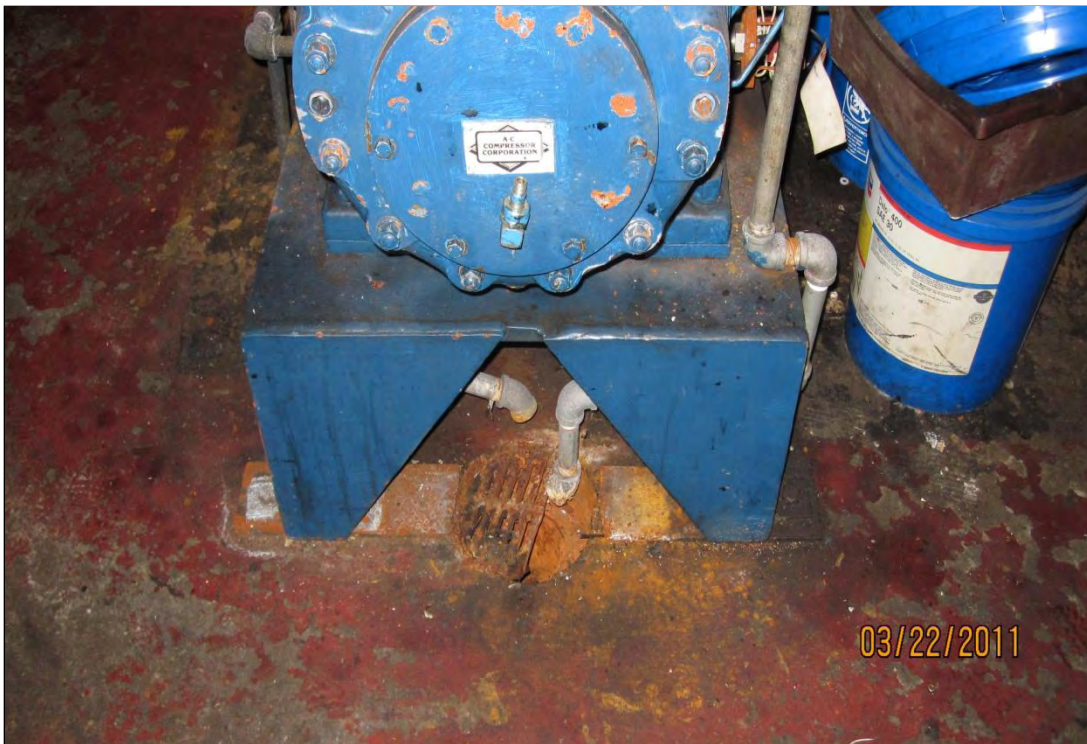
Photo 28. Floor drain located inside the engine room building. The drain is located below an ammonia compressor. Source of pipes directed towards the drain was not determined.
