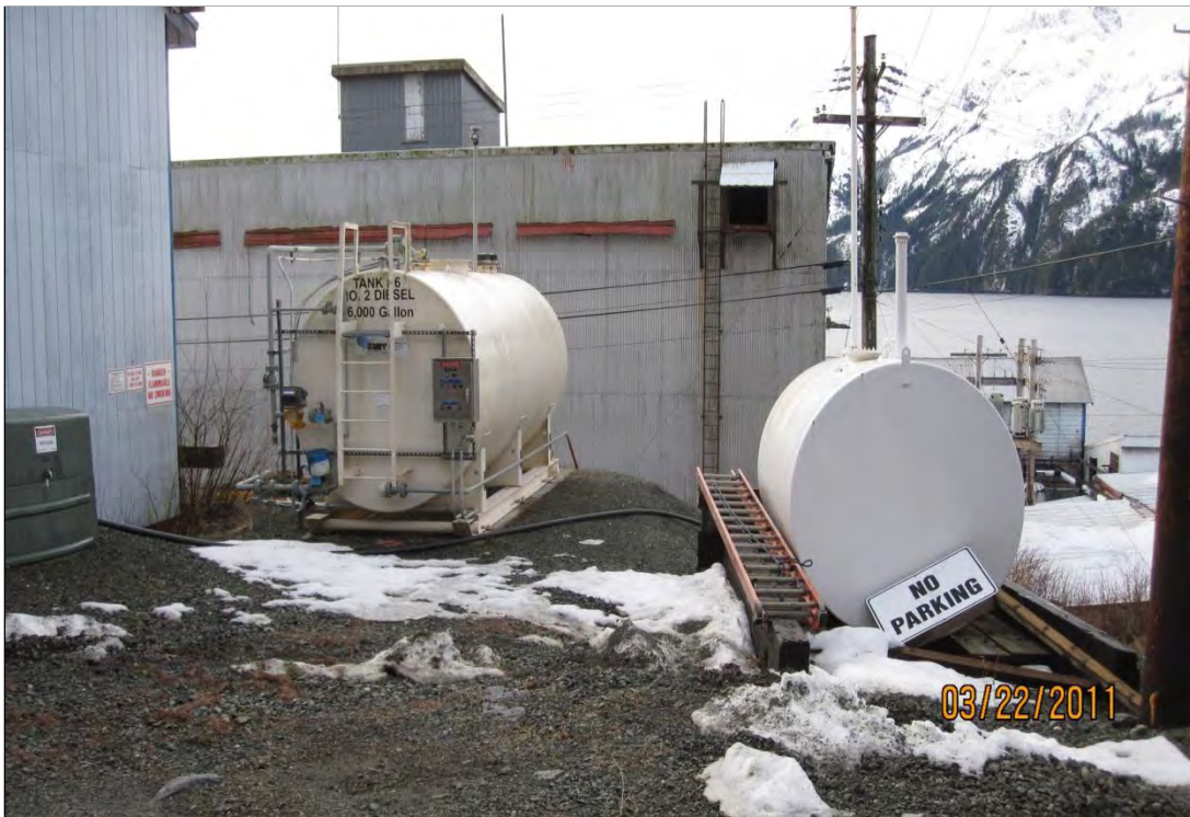
Photo 18. Power module. One of two (west most) power module 6,000 gallon ASTs, and smaller non-compliant (unplumbed) single wall AST on right side of photo.
