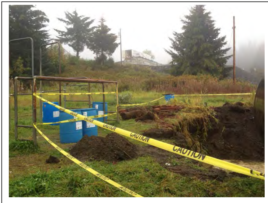
Photo 6: Impacted soil stockpile and drums of residual heating oil removed from the tank prior to excavation; looking north. (September 17, 2014)
