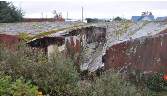
Figure 12. Overview of the collapsed roof of the first addition, right of image, with second addition on left; view to the south (©TNSDS 2014).
