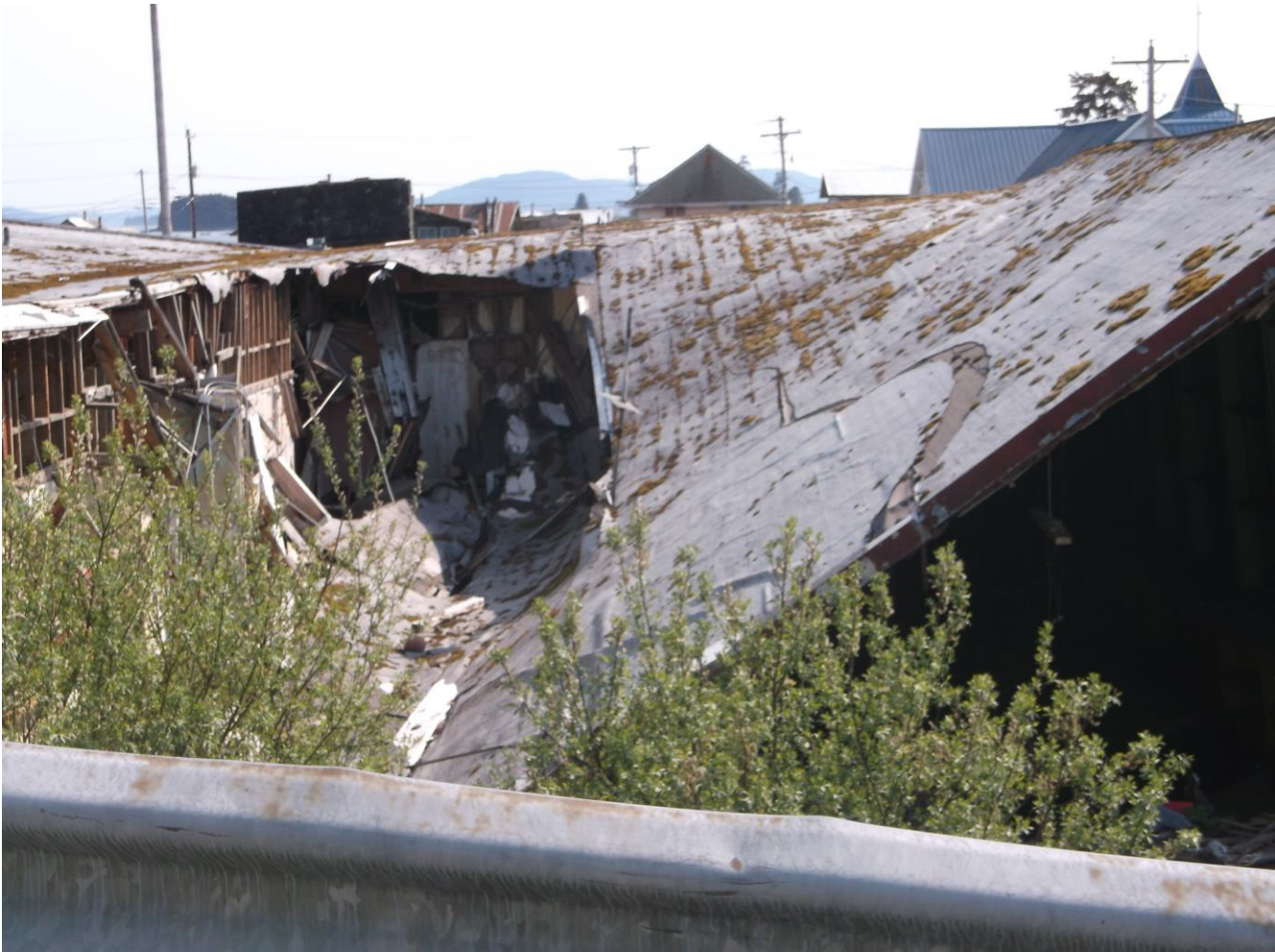
Figure 3: The collapsed roof of the School.
