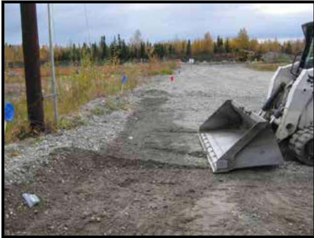
Photo 31: 9/22/2011 – Typical surface stain corrective action.
