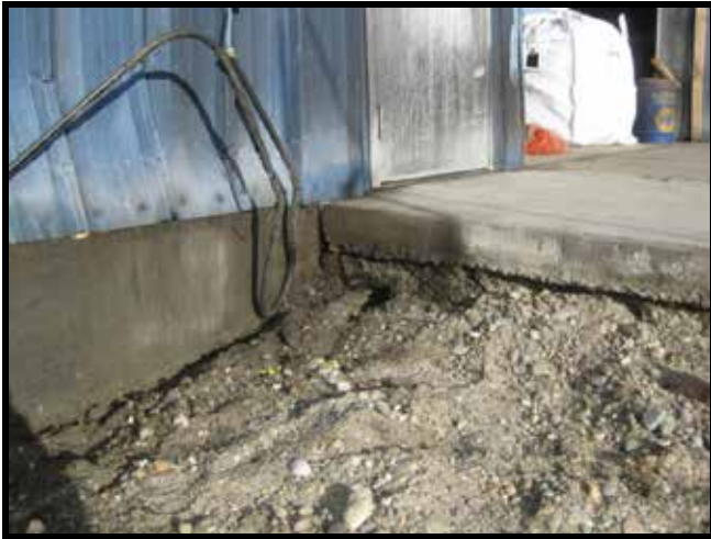
Photo 37: 10/6/2011 – Surface impacts from oily sludge at southern overhead door.
