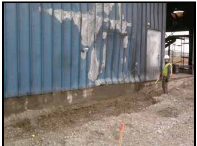
Photo 42: 10/12/2011 – Visible stained soils remaining within structural prism.
