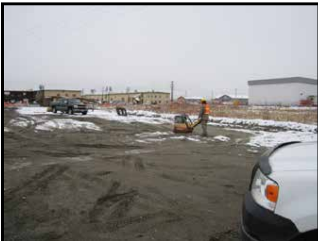
Photo 59: 10/17/2011 - Typical site-wide backfill and compaction to return pits and other areas to previous grade.
