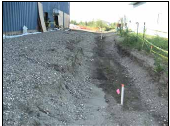
Photo 18: 7/6/2011 – West Ditch after initial excavation and installation of monitoring wells (MW2 in foreground).
