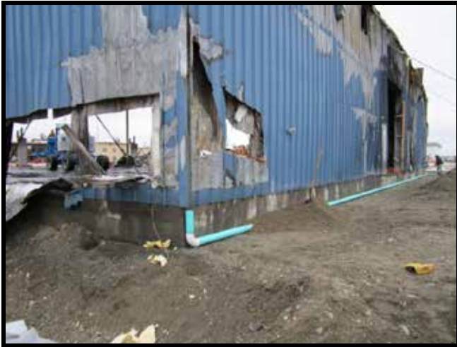
Photo 55: 10/17/2011 – Vapor extraction and bedding gravel across the south end of the building.
