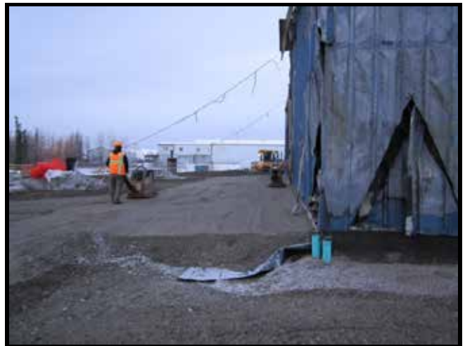
Photo 58: 10/18/2011 – Backfill and 95% compaction above the vapor barrier on the south side of the building.
