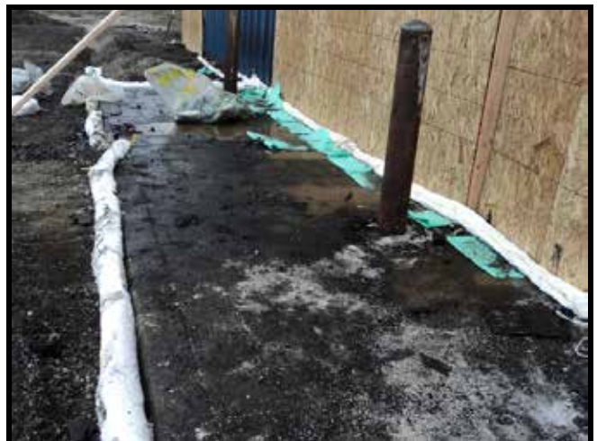
Photo 6: 5/27/2011 – East warehouse door sludge containment.
