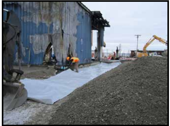
Photo 56: 10/18/2011 - Typical vapor barrier installation above piping on the eastern side of the building.
