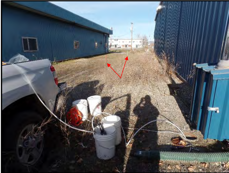
Photo 1: October 9, 2018. Looking north along the west side ditch during sampling of MW3 adjacent to the vapor extraction system (VES) housing and stack. MW1 and MW2 (white stickup) are located (red arrows) in the ditch at the property boundary.
