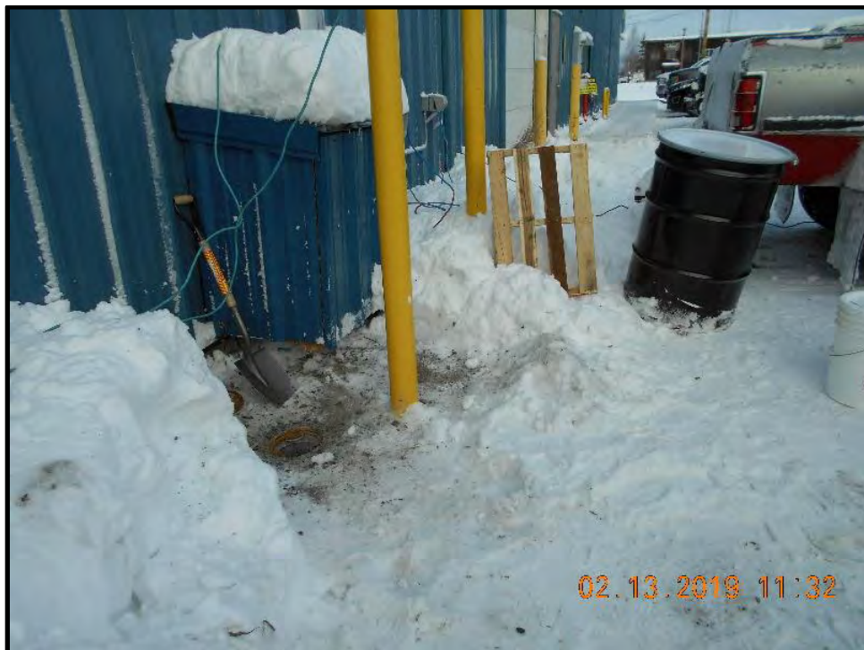
Photo 4: February 13, 2019. Looking north during sampling of MW4 located adjacent to the east side VES housing.
