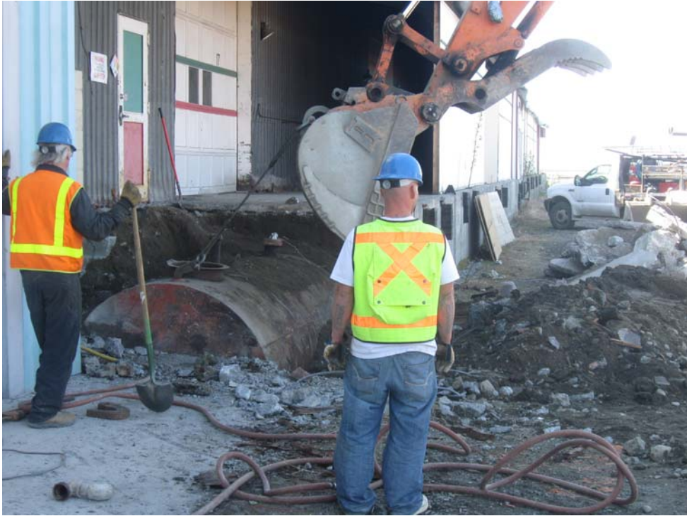
Photograph 1: Concrete walls removed and underground storage tank (UST) ready for removal. View looking west
