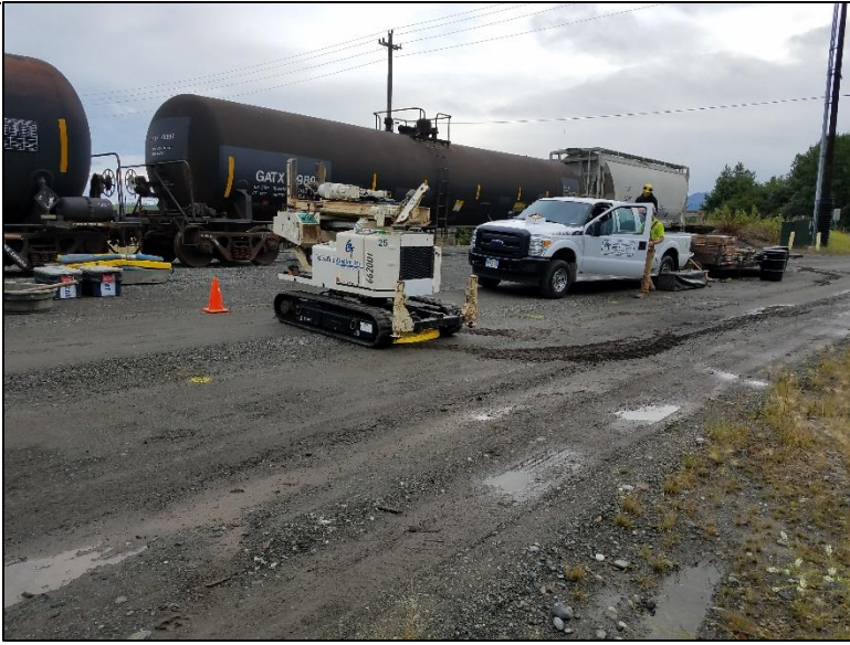
Rig mobilizing to North UST area. Yellow marks indicate natural gas line. Facing northeast.
