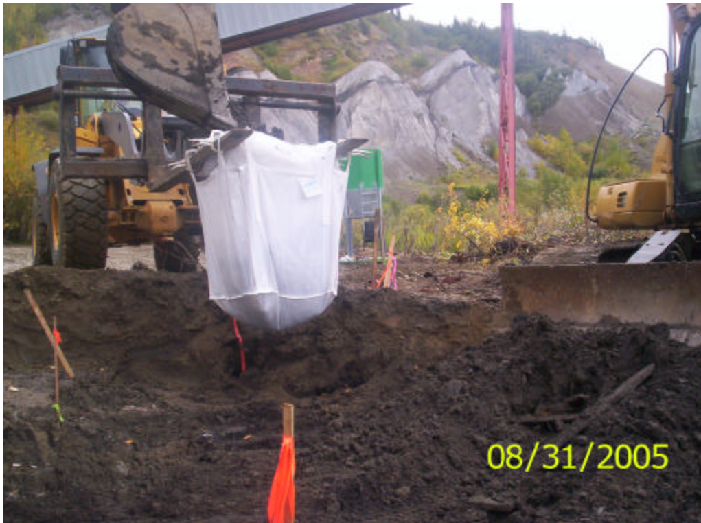
Photo 6. Loading supersacks with contaminated soil directly out of the ground. Notice conveyor structure in background. Bearing of picture is nearly due east.
