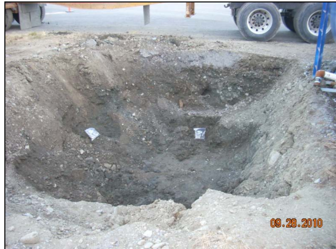
Photo 8: Excavation after filling second truck, with screening samples at sample locations, looking south.
