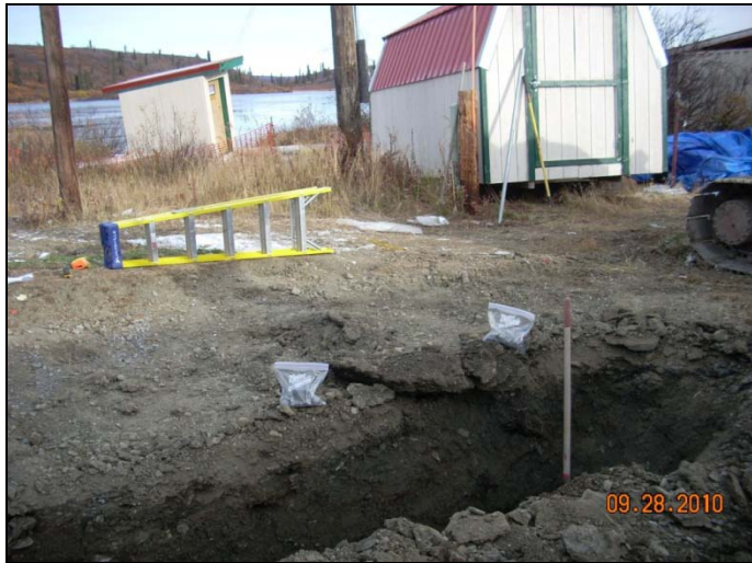
Photo 5: Water intake structure at lake edge and shed temporarily moved for excavation, with initial trench and screening samples, looking north.
