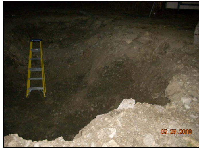
Photo 12: Excavation after removing and stockpiling contaminated material from the east wall, looking north.
