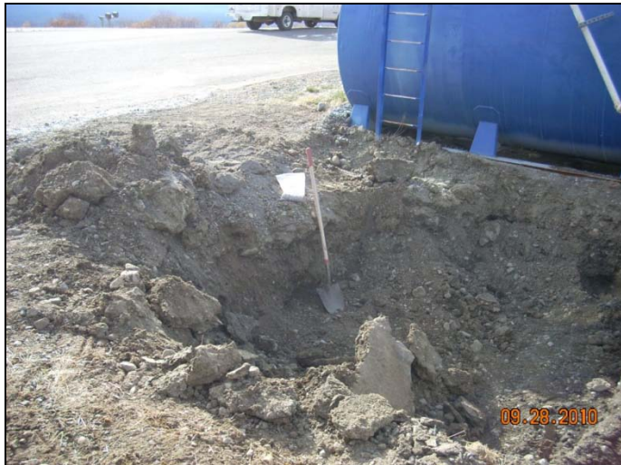
Photo 7: Excavation after filling first truck and screening sample location at shovel tip, looking southwest.
