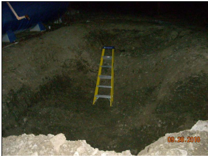
Photo 11: Excavation after removing and stockpiling contaminated material from the east wall, looking north.
