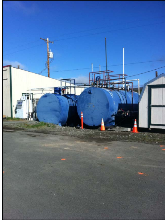
PHOTOGRAPH 3: CLOSER VIEW OF THE SOUTHERN PORTION OF THE ASTS, LOOKING NORTHWEST (JUNE 2011)
