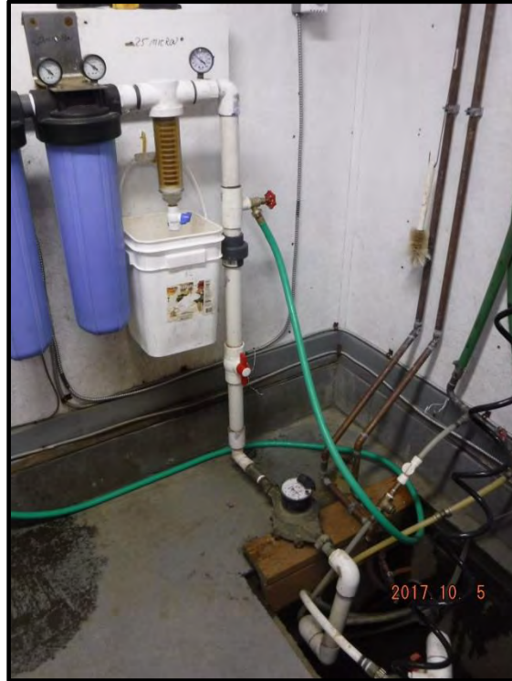
Photograph 11: Inside of well house, PVC pipe leads from drinking water well to filtration system and the drinking water storage tanks. Once the system was purged, the sample was collected prior to the filters.
