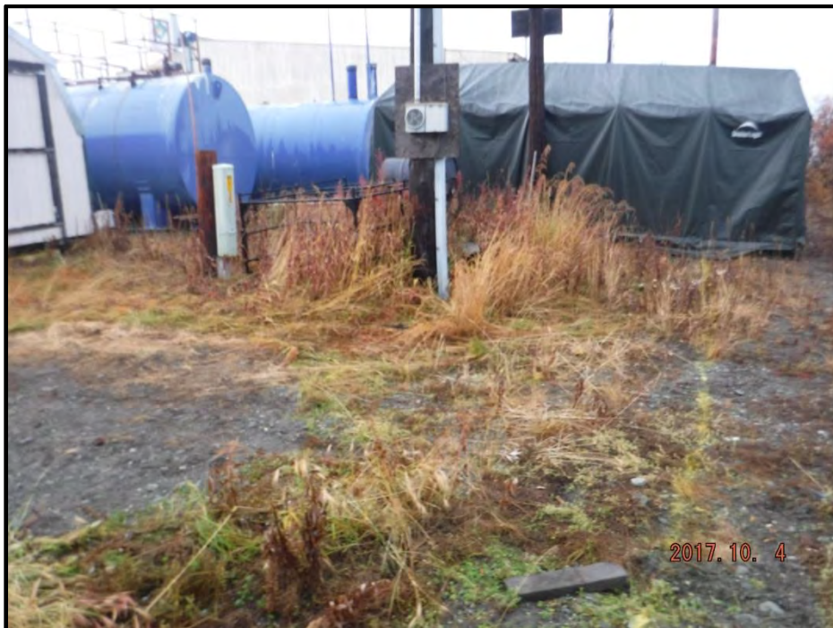
Photograph 4: Water Line drawn in yellow marking paint by site owner's son extends to the west, directly north of the fuel tanks.
