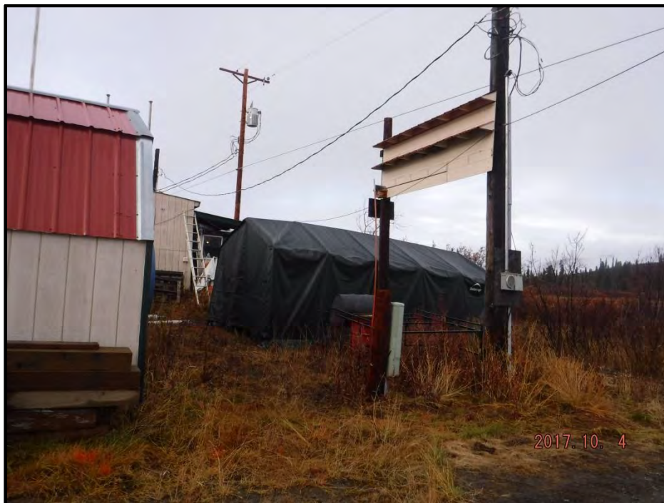
Photograph 2: Communication Utility Box and Utility Corridor located directly north of the fuel tanks and south of the Unnamed Lake. Picture was taken facing west.
