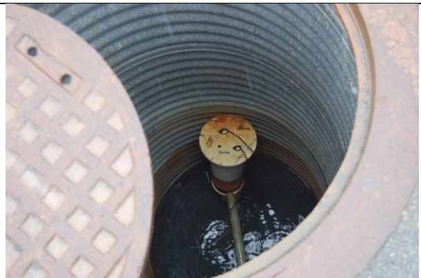
Inside BH1. Cap damaged and immovable.
