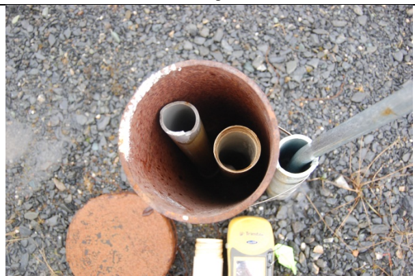
Inside damaged MW1.
