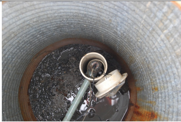
MW4 highlighting the pump system.
