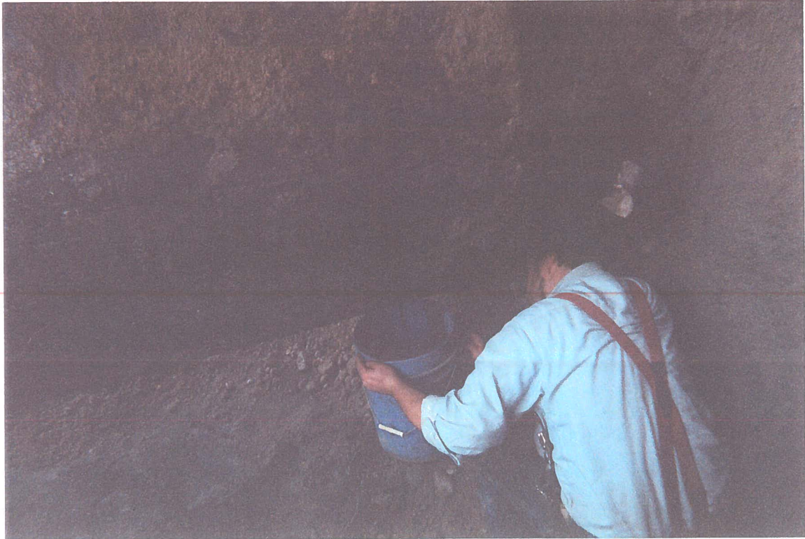
A Channel Construction worker uses a bucket to catch fuel leaking from the UST.
