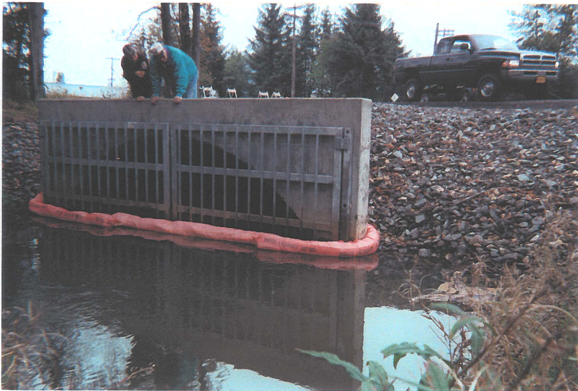
ADEC and USF&WS personnel inspect sorbent boom in Duck Creek at Cessna Dr culvert.
