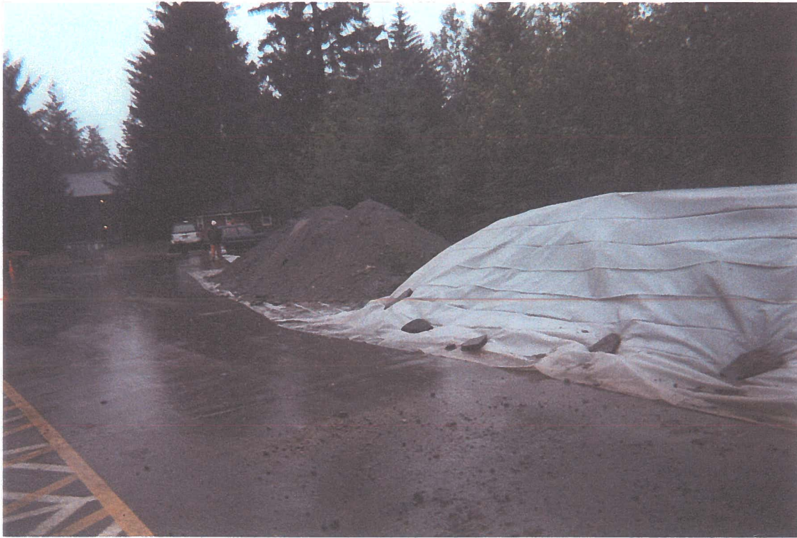
Contaminated soil stockpile in the Travelodge parking lot.
