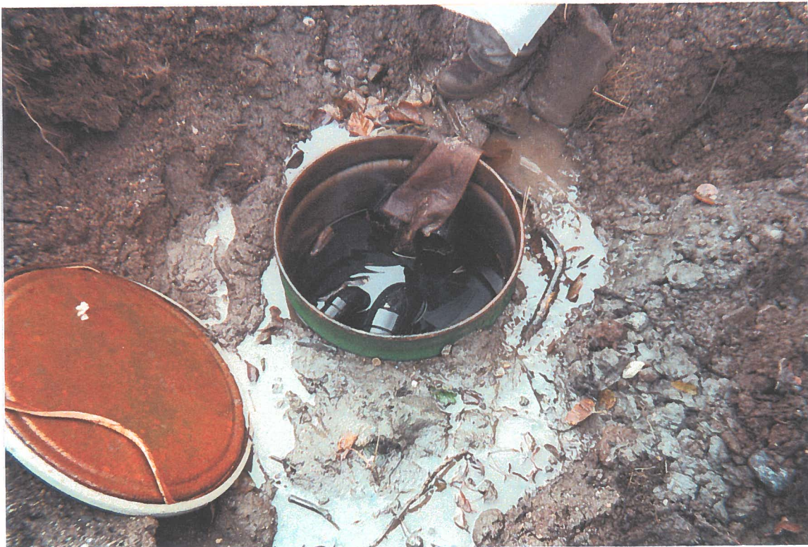
Oil/water separator, late September 2000.
