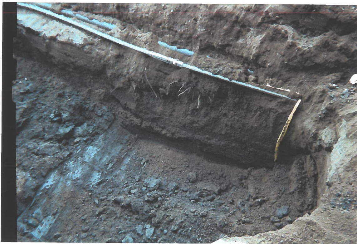
Blue silt at the bottom of the Travelodge excavation prevented the spread of diesel contamination to the water table.
