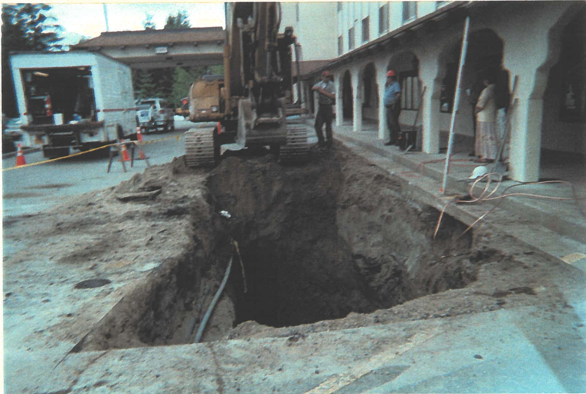
Channel Construction removed the UST from the west side of the Travelodge, June 7, 2001.
