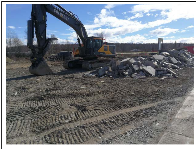
Photo 4: Looking northwest during removal of the floor slab. (April 8, 2019 – photo provided by Coldfoot)
