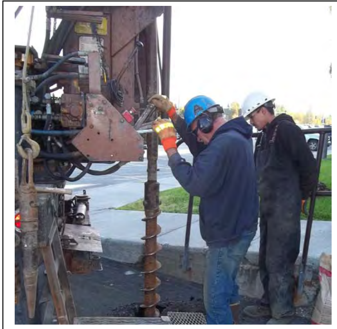
Photo 7: An auger was advanced down to 5 feet bgs to re-open the collapsed hole of Well B7MW. Bentonite chips were backfilled while the auger was retracted. (September 16, 2013)
