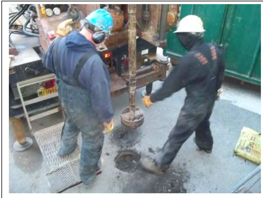
Photo 1: Discovery making two asphalt cuts in an attempt to locate Well B6MW. (September 16, 2013)
