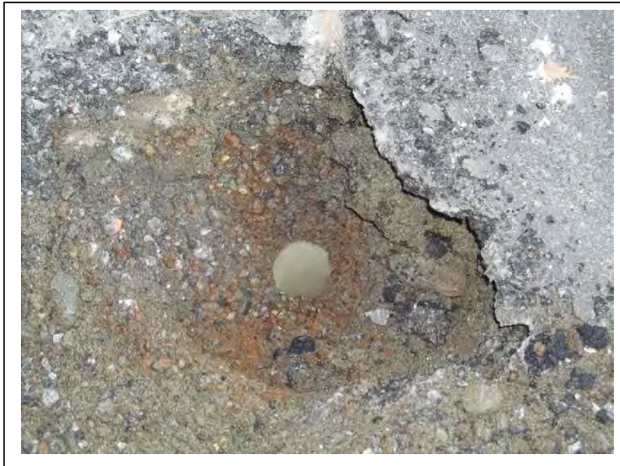
Photo 3: Well B7MW casing after damaged monument sleeve was removed. (September 16, 2013)
