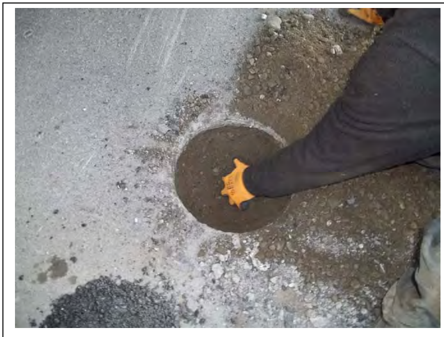
Photo 2: Discovery hand-dug down to approximately 6 inches bgs to locate casings of Wells B4MW, B5MW, B6MW and B7MW. (September 16, 2013)
