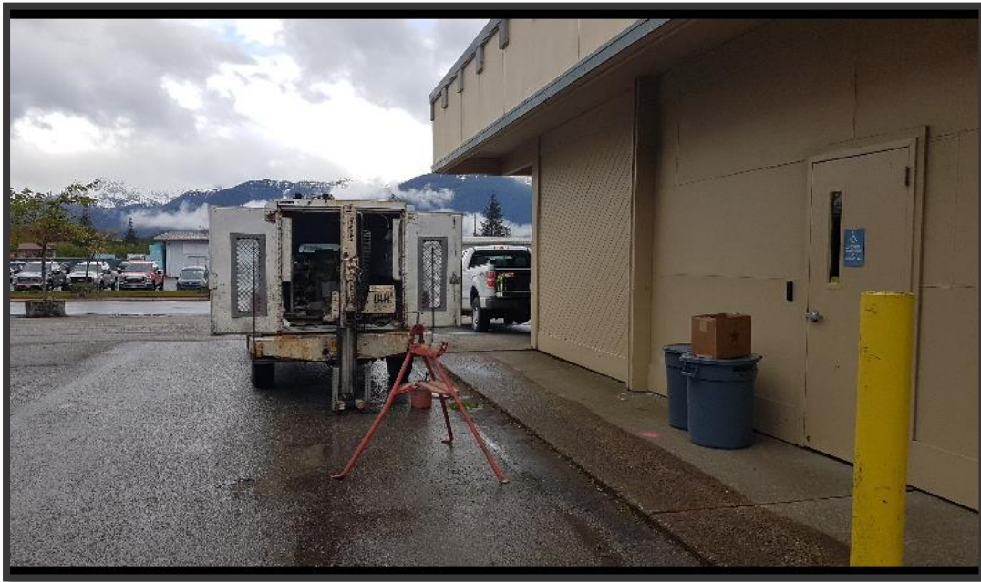
Photo 1: View looking south at the location for BH-01/MW-1. Soil sampling and monitoring well installation was performed with a Geoprobe GH42 direct push truck mounted rig, seen in photo.
