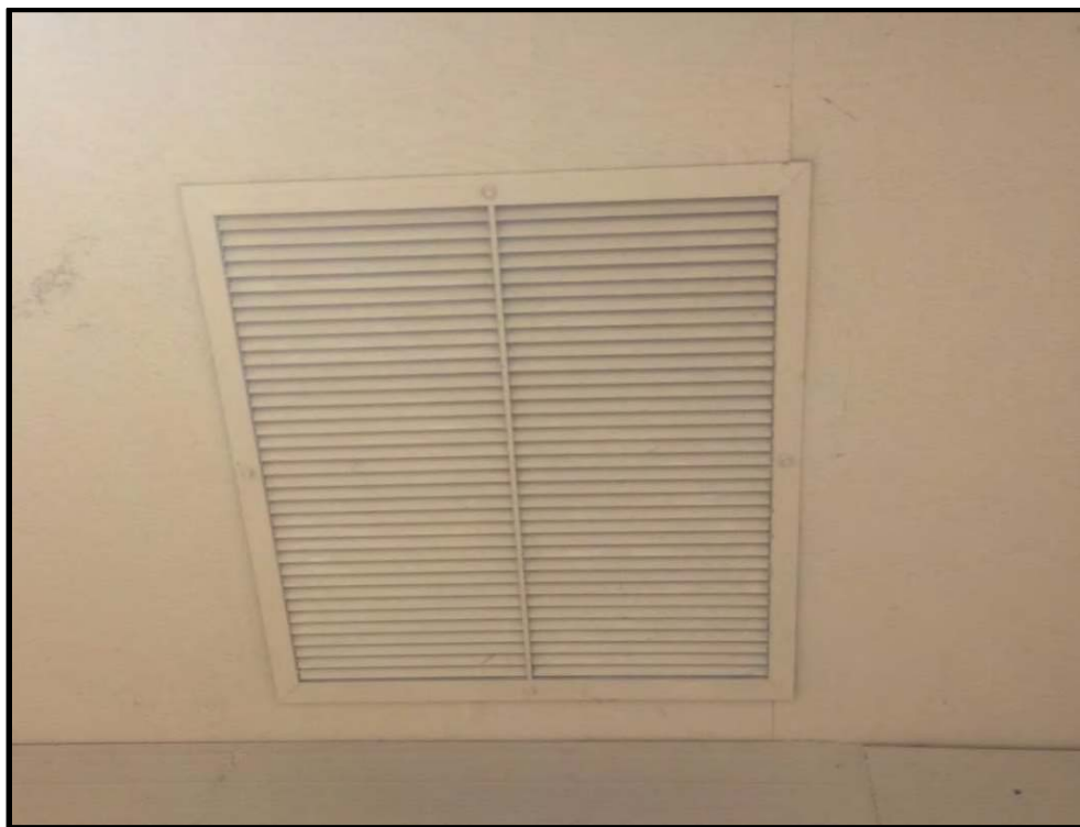
Photo 2: One of several fresh air intakes into the plenum of the building.
