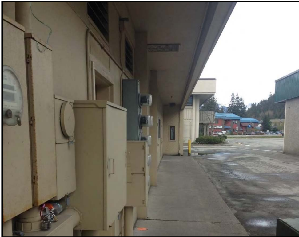
Photo 3: Looking north along east side of the building. Summa canister 5xxB is at the lower left corner of the photo. Upper center edge of the photo shows the two main fresh air intakes, in the wall, for the two diesel fueled HVAC systems.
