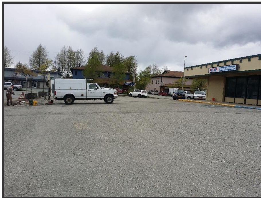
Photo 6: Drill rig set up at location BH-4 on south side of the parking lot.
