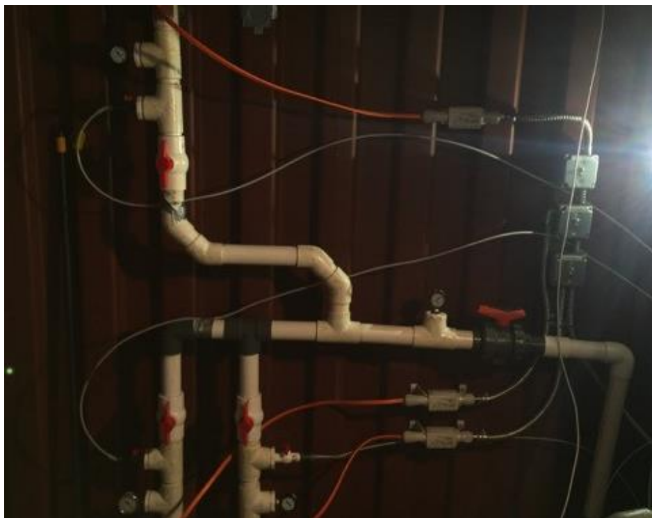
SVE system: Three collection pipes entering manifold to blower
