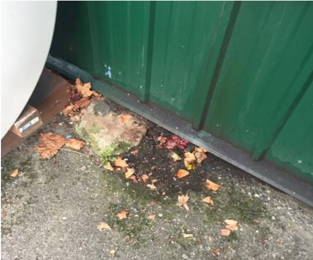
Staining from pipe from AST into asphalt
