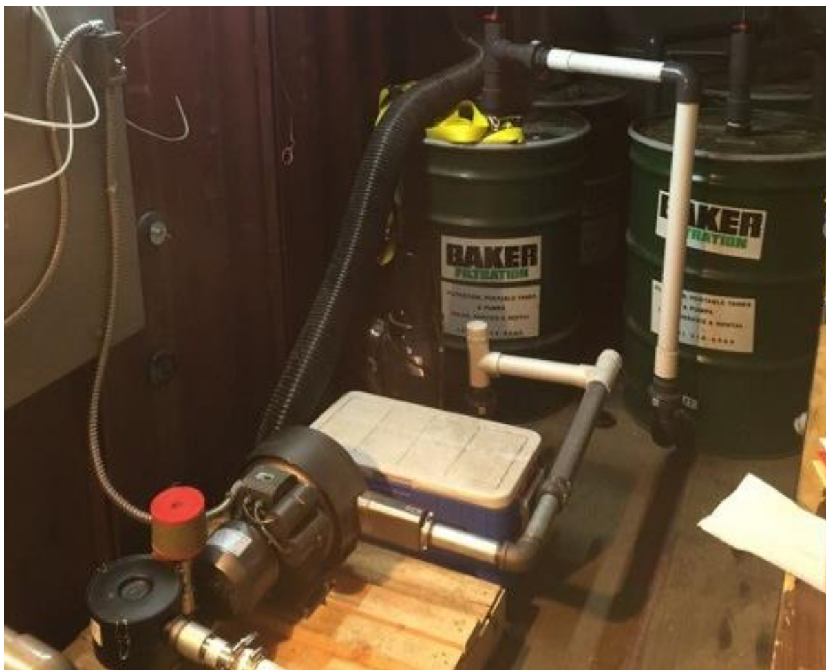
SVE system: Blower with granulated activated carbon containers
