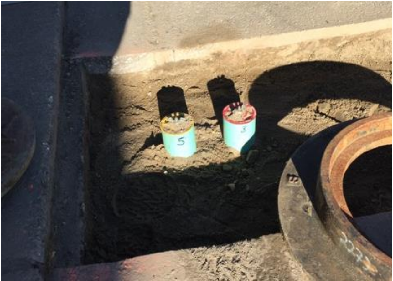
Termination of SVE trench collection piping
