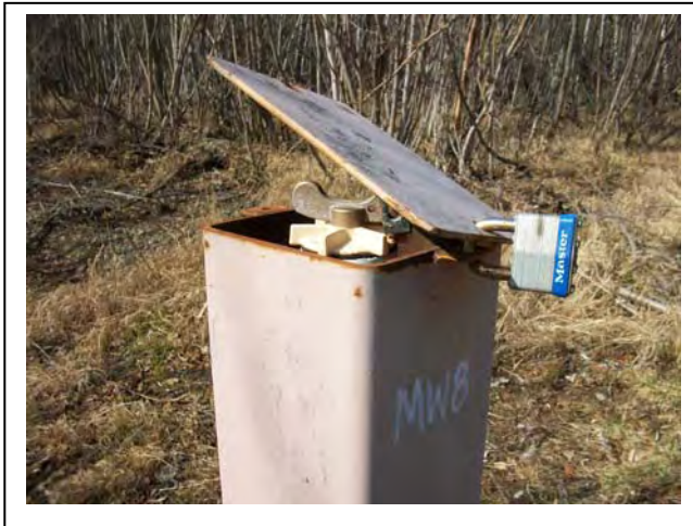
Photo 3: Wells such as RA-MW-8 were frost-jacked and needed to have their PVC risers cut to close the casing. (5/18/2010)
