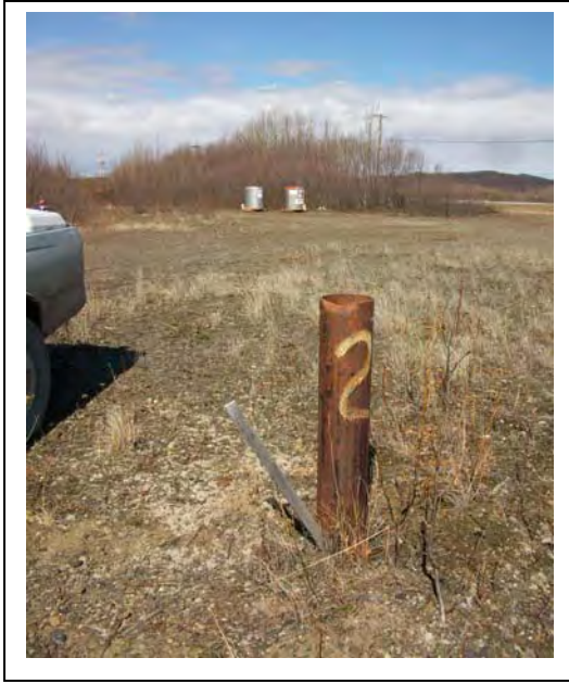
Photo 1: Looking northwest, the Runway Apron drinking water well casing was damaged, and did not have a top closure. (5/17/2010)
