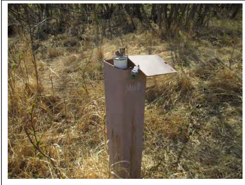
Photo 5: Looking south, frost jacking at Monitoring Well RA-MW8 at the Runway Apron area. (5/13/2014)
