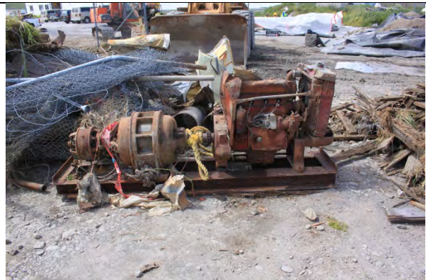
Generator and motor removed. Motor appeared to contain no fluids.
