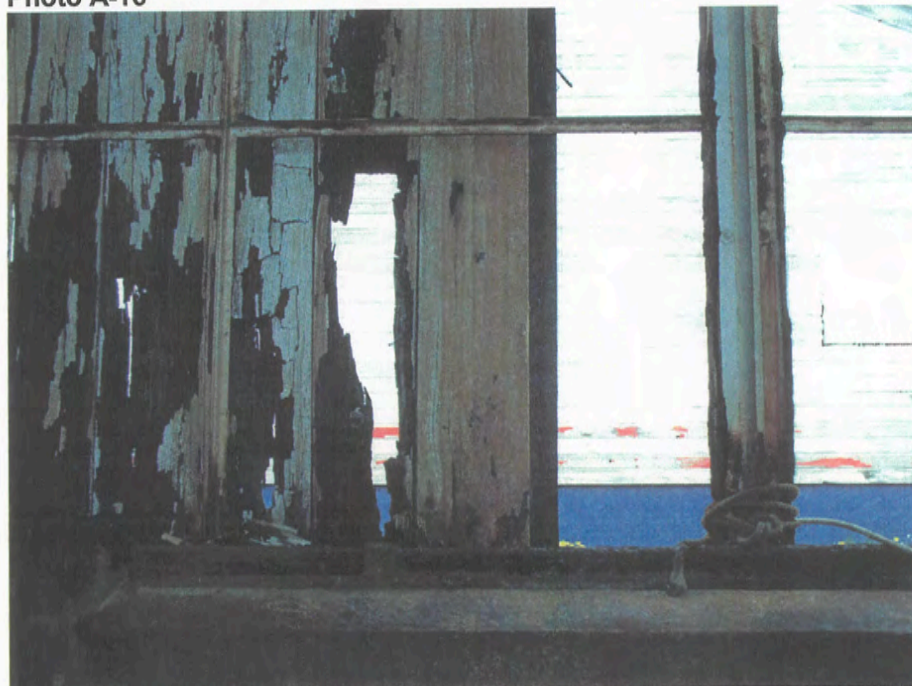
North elevation detail, looking through metal sash window frames to exterior wood decking of Room 106-Torpedo Rack, June 2003
