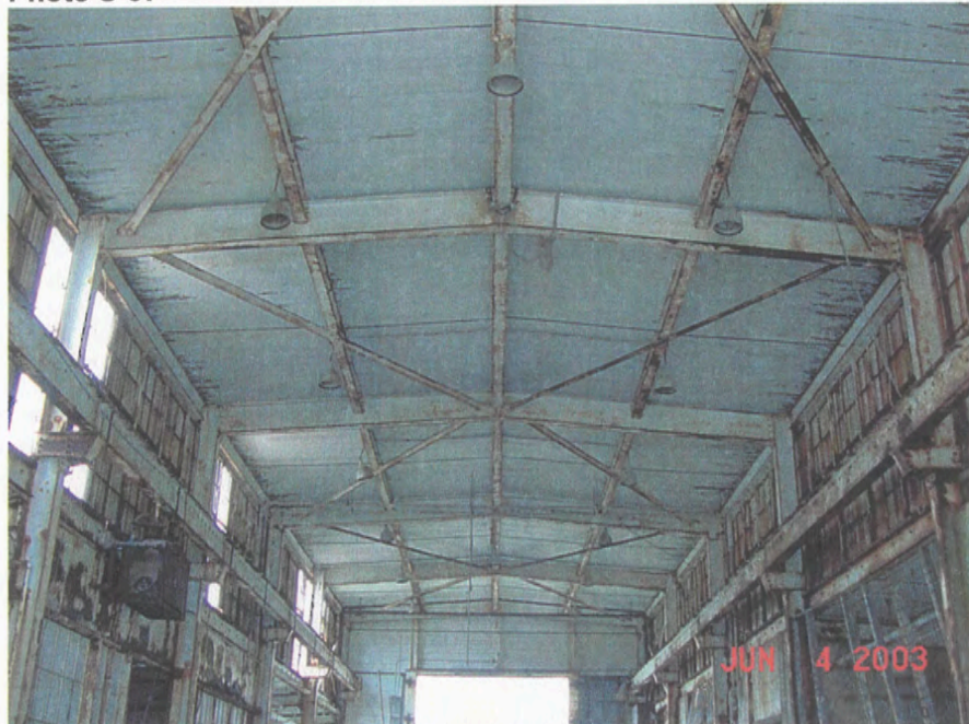
Grid 1-7/B-C – interior elevation high central roof, horizontal roof bracing looking west, June 2003
