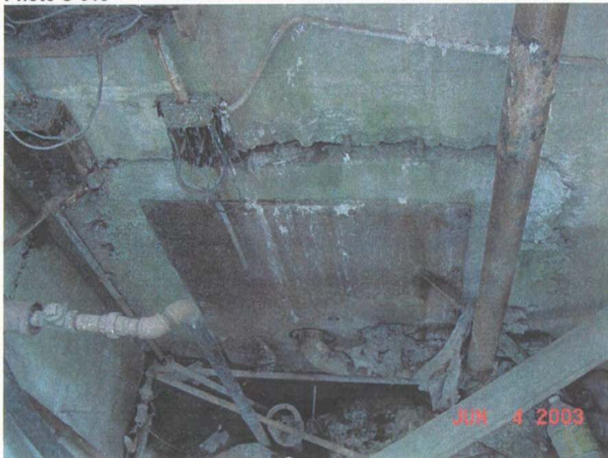
Grid 2.5/D – pit, hole through outside wall below outside grade, patched, June 2003
