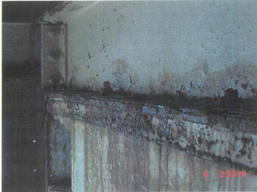
Grid 6/D – Channel over top of interior concrete wall, typical W girder above, June 2003
