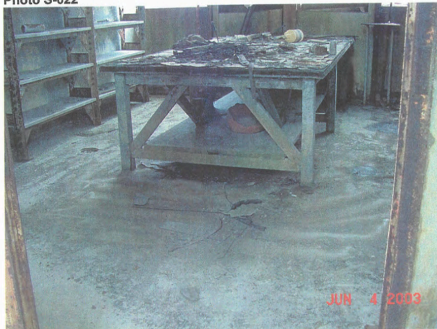
Grid 3-4/C-D – east floor drain, delam/grade away from bottom of slab on grade, June 2003
