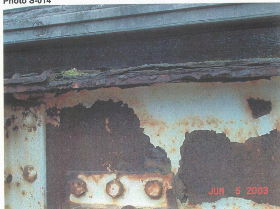
Grid 7/C – top of east girder, misc. steel between girder and roof deck, June 2003
