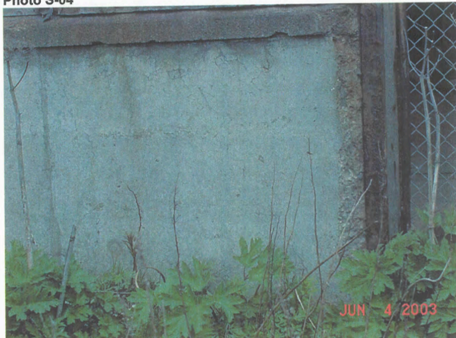
Grid 1/C – exterior concrete wall, damaged corner , June 2003
