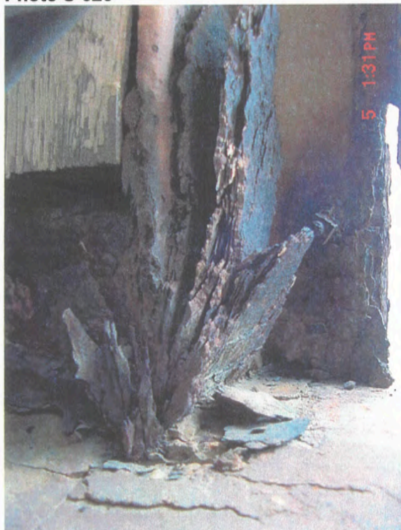
Grid 7/A.5 – Steel angle, jamb north side of parachute loft, east windows, June 2003
