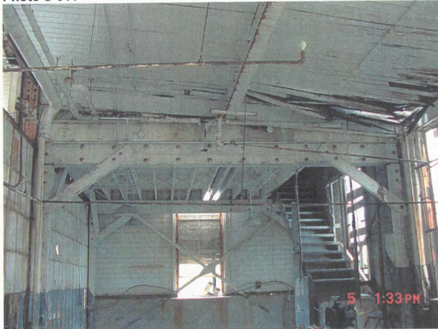
Grid 7/A-B – interior elevation, vertical cross bracing parachute loft below intermediate floor, June 2003
