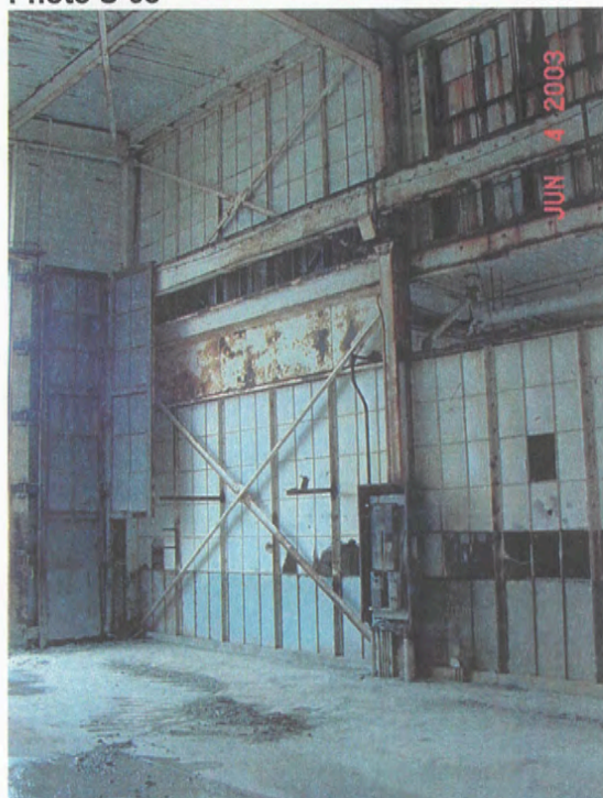
Grid 6-7/B – interior elevation, vertical cross bracing high central roof to SOG , June 2003
