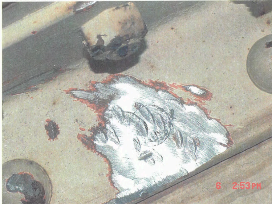
Grid 6/C.6 – Head of rivet ground off to face of W beam web, June 2003
