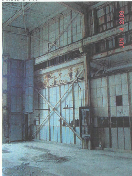
Grid 1-2/C – interior elevation, cross bracing high central roof to low side shed roof, June 2003
