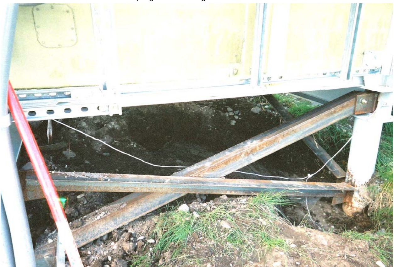
Completed excavation beneath generator module, note liner at base of excavation. Looking west.
