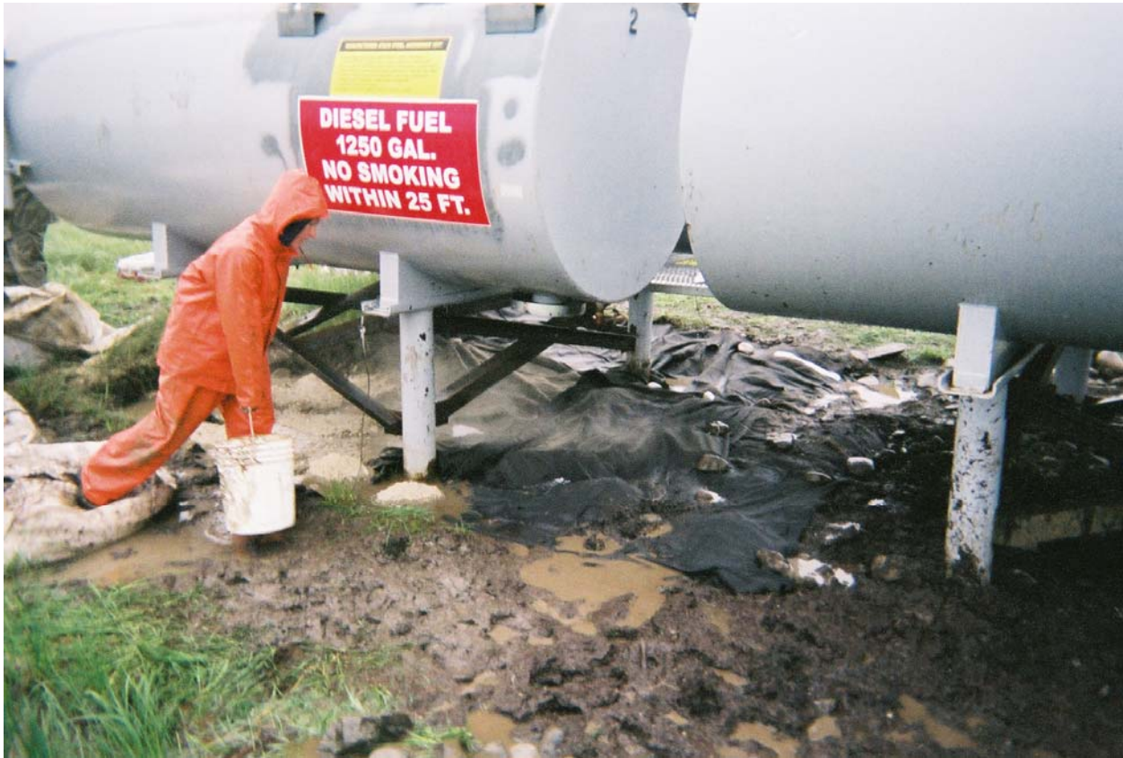
Geofabric liner beneath ASTs 2 and 3, ready for base layer of D-1 fill. Looking southeast.
