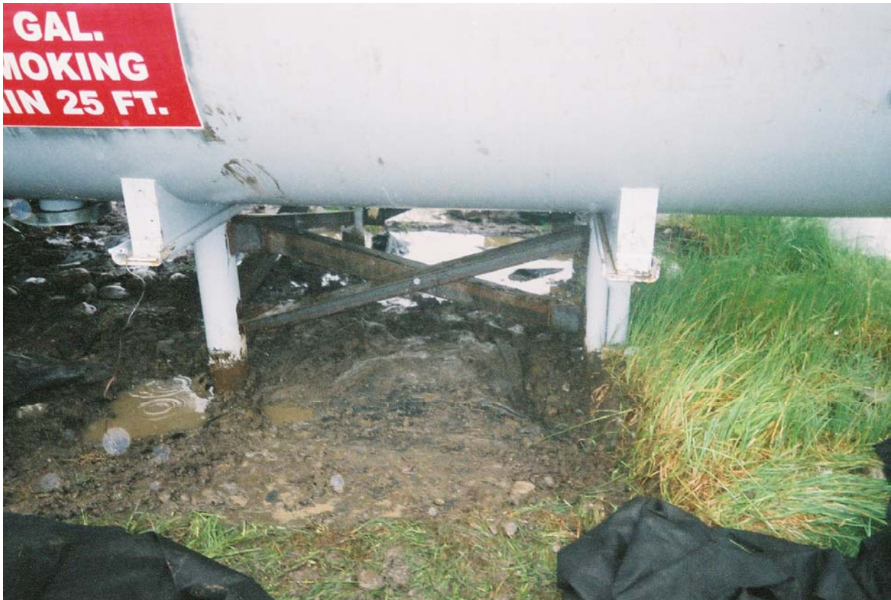
Finished excavation beneath AST 3, note liner at depth of excavation. Looking north.
