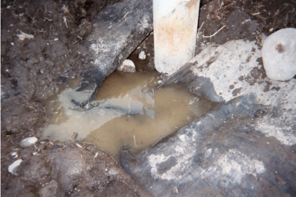
Sheen on water in excavation beneath Tank 1.
