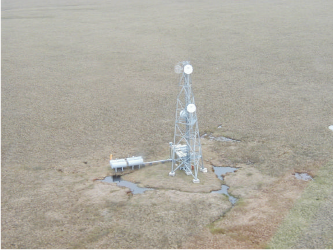
Aerial view of Costa Hill Repeater Site, looking south.
