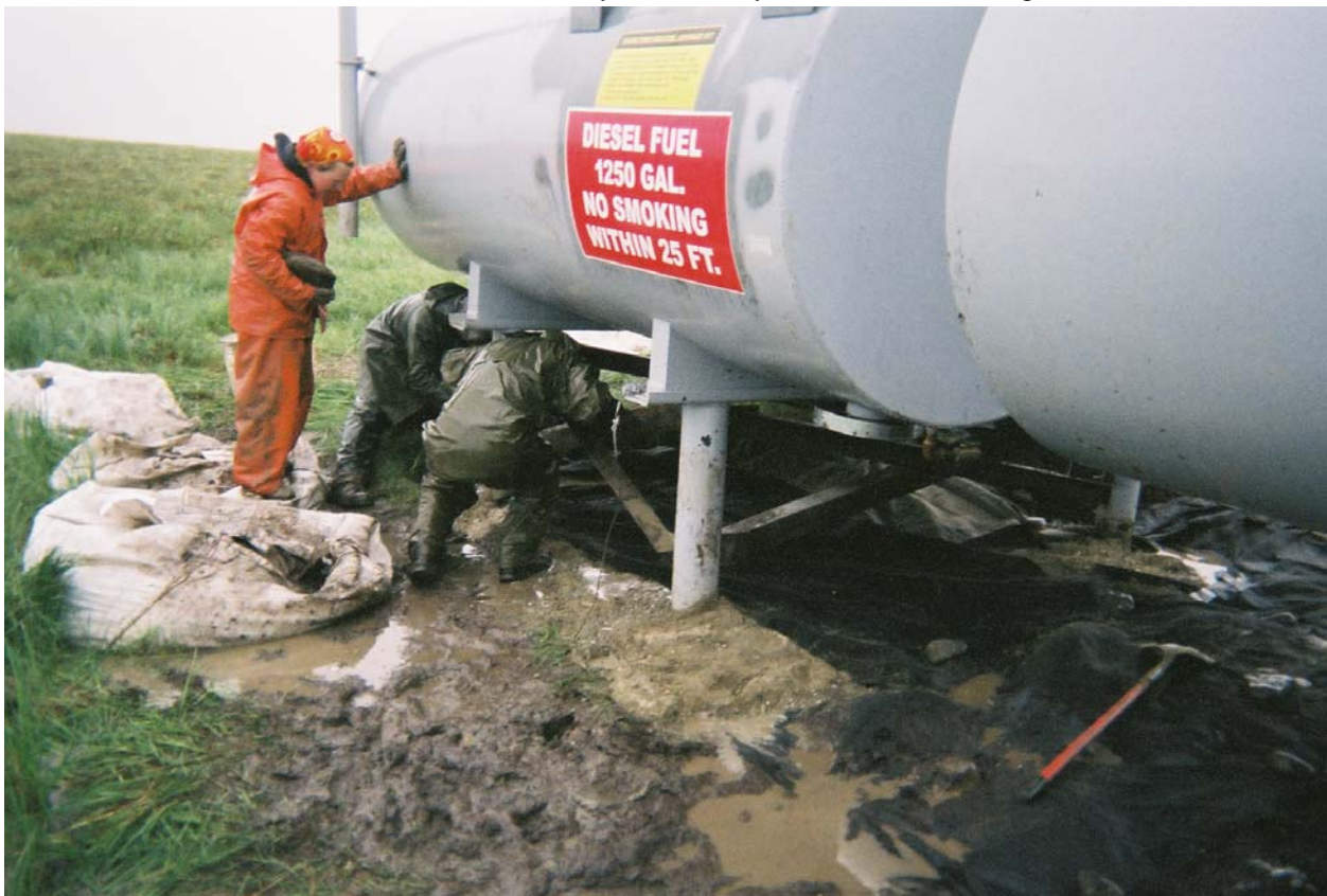
Applying geofabric liner on top of D-1 fill, preparing to complete backfill with native material. Looking southeast.
