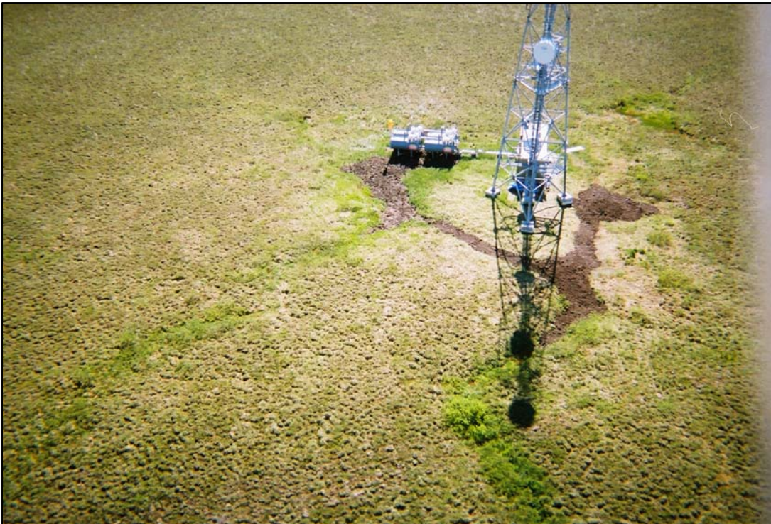
Aerial view of Costa Hill Repeater site after all dewatering and backfill activities complete.
