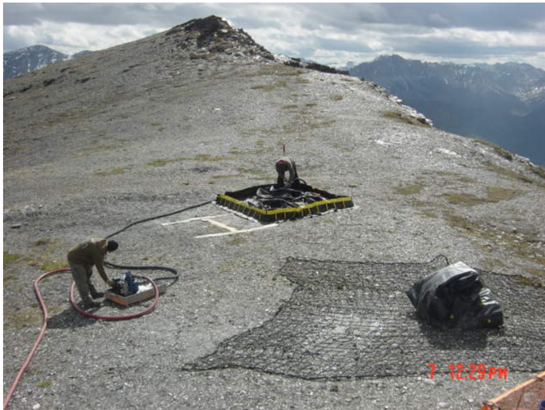
Pump fuel from bladder in secondary containment via modular portable pump with secondary containment.
