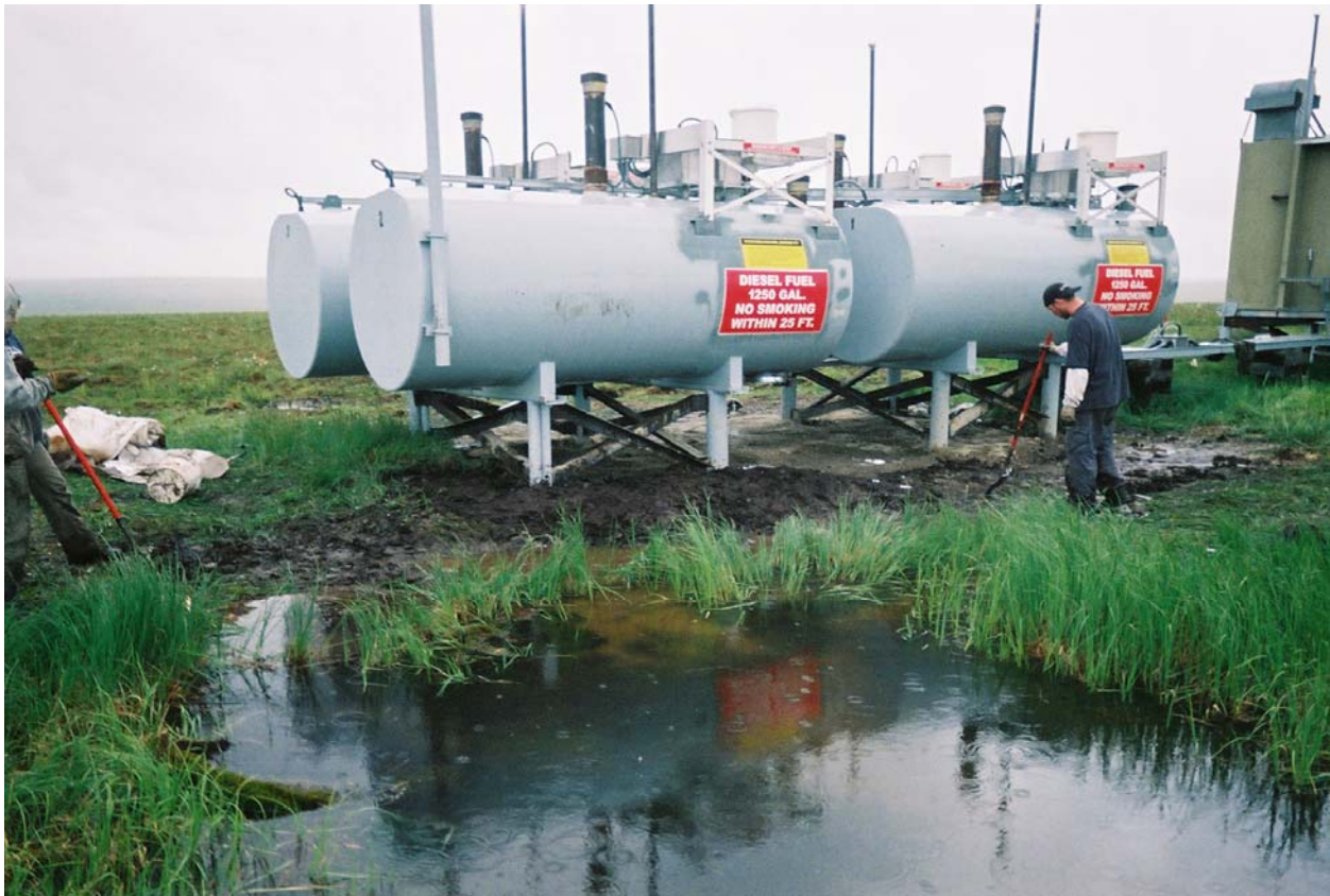
Completed backfill at ASTs with dike of native material between AST 1 and surface water. Looking southwest.
