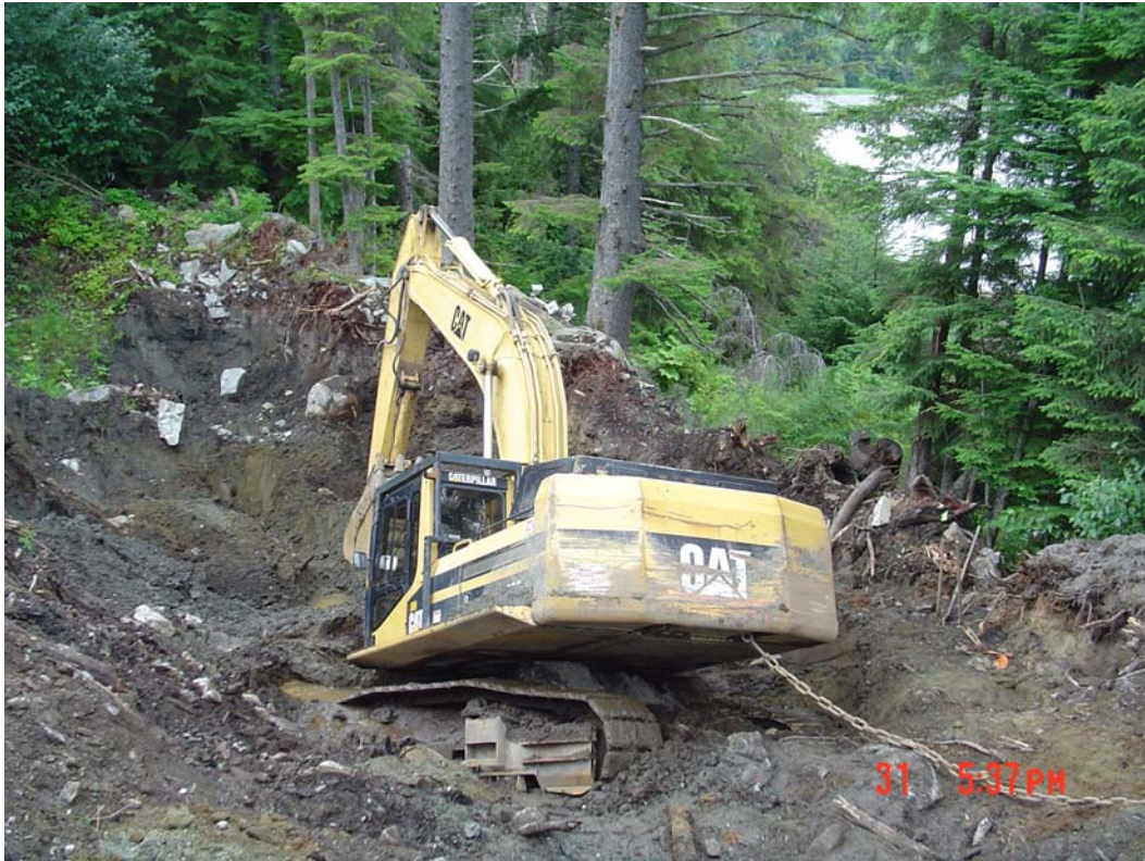
Photo 10. Excavator Stuck In Bottom of Excavation
