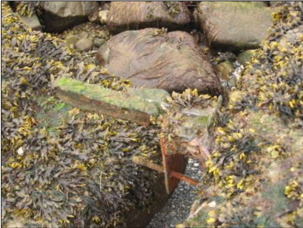
Photograph 13. Example of metal removed at the Seaplane Ramp.
