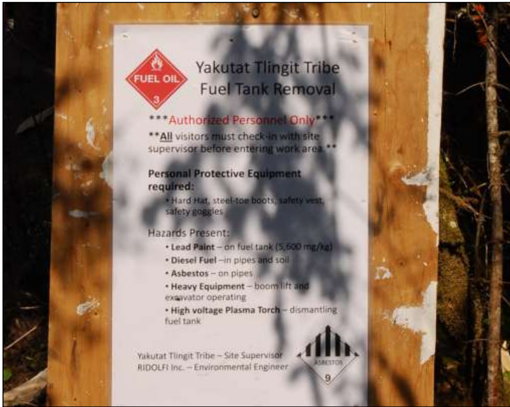
Photograph 1. Warning Sign: Fuel Tank Removal and Asbestos Work
