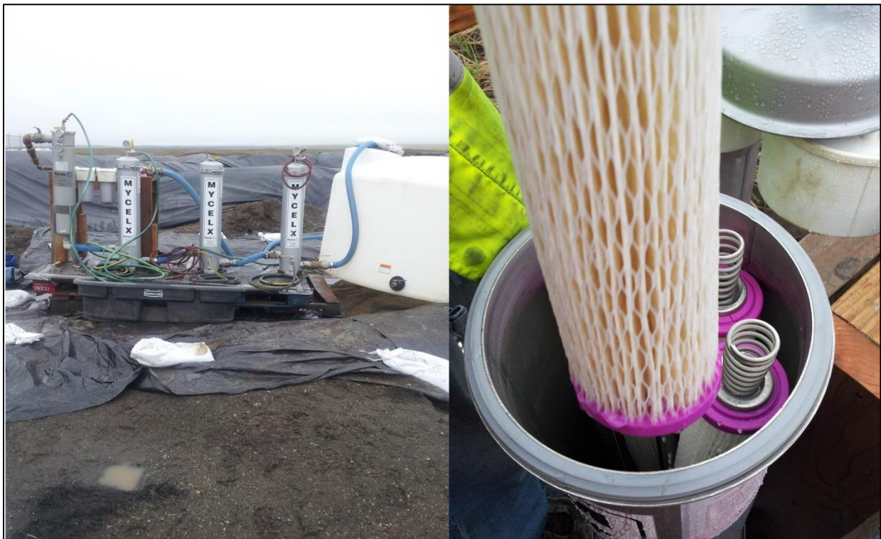
Figure 14. MYCLEX filtration system in operation at Port Heiden Community landfill, showing detail of the filter.
