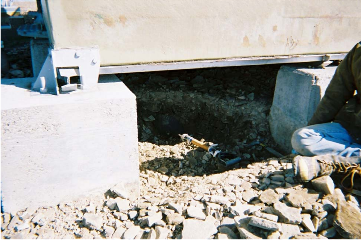
Completed excavation beneath northwest corner of the Generator Module with shovel for scale.
