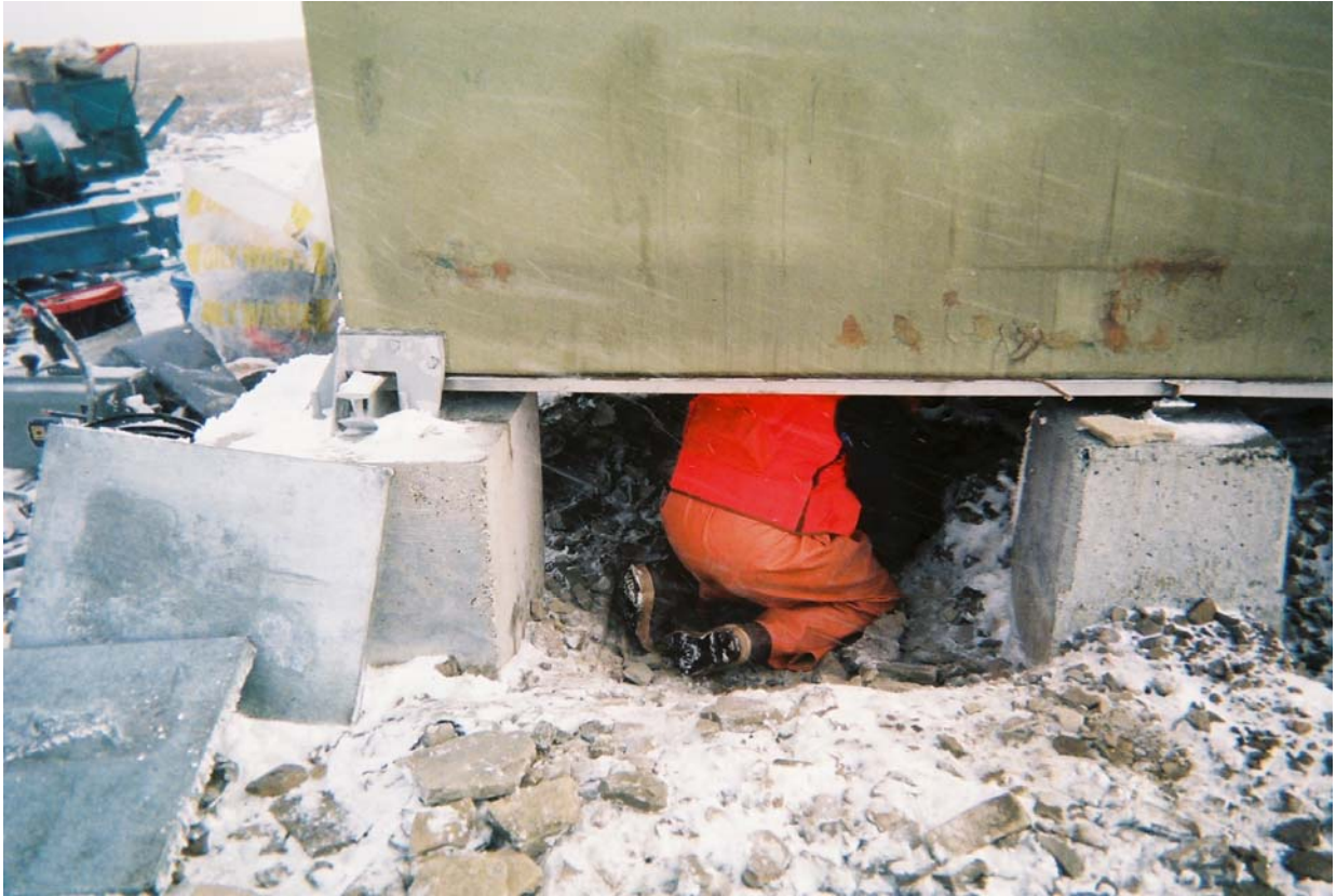
Collecting confirmation samples from the completed excavation beneath northwest corner of the Generator Module.
