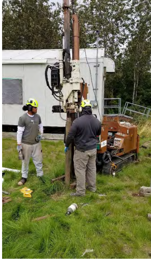
Photo No. 1 – 26 August 2019 Drillers work to advance the boring for MW2A. View facing North.
