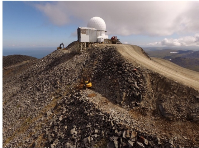
Figure 1-3. Site SS016, note the excavator and the steepness of SS016.
