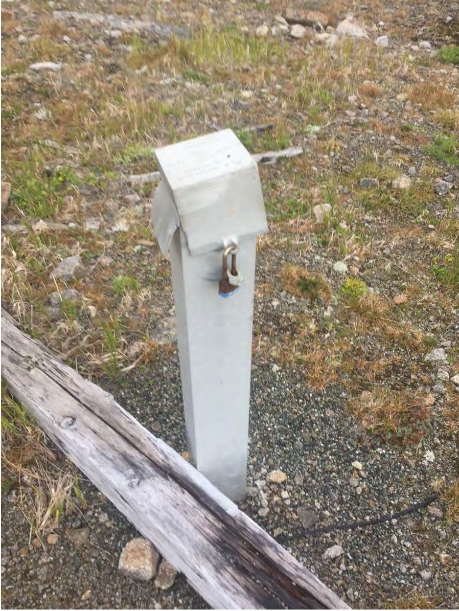
Site SS015. WW03 close-up.
