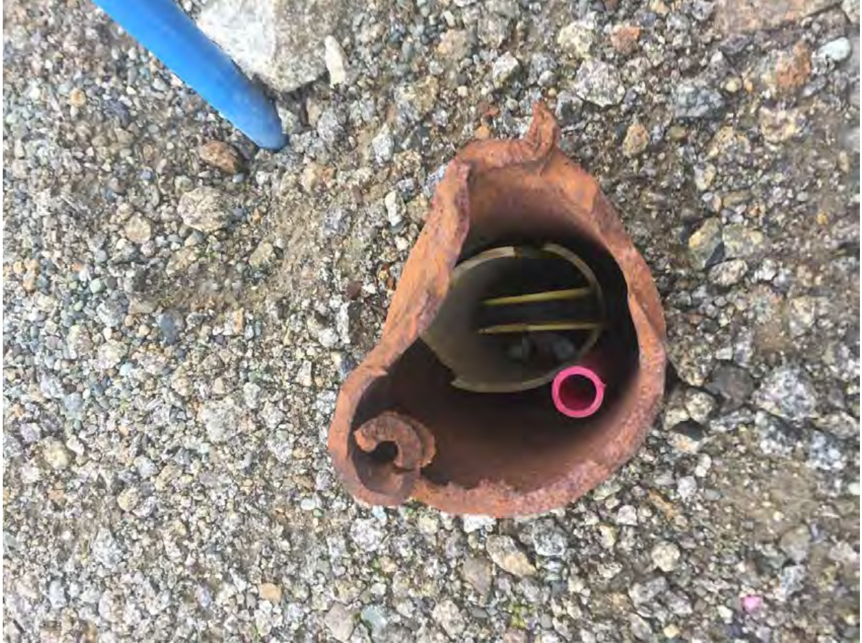
Site SS015. WW01 close-up.
