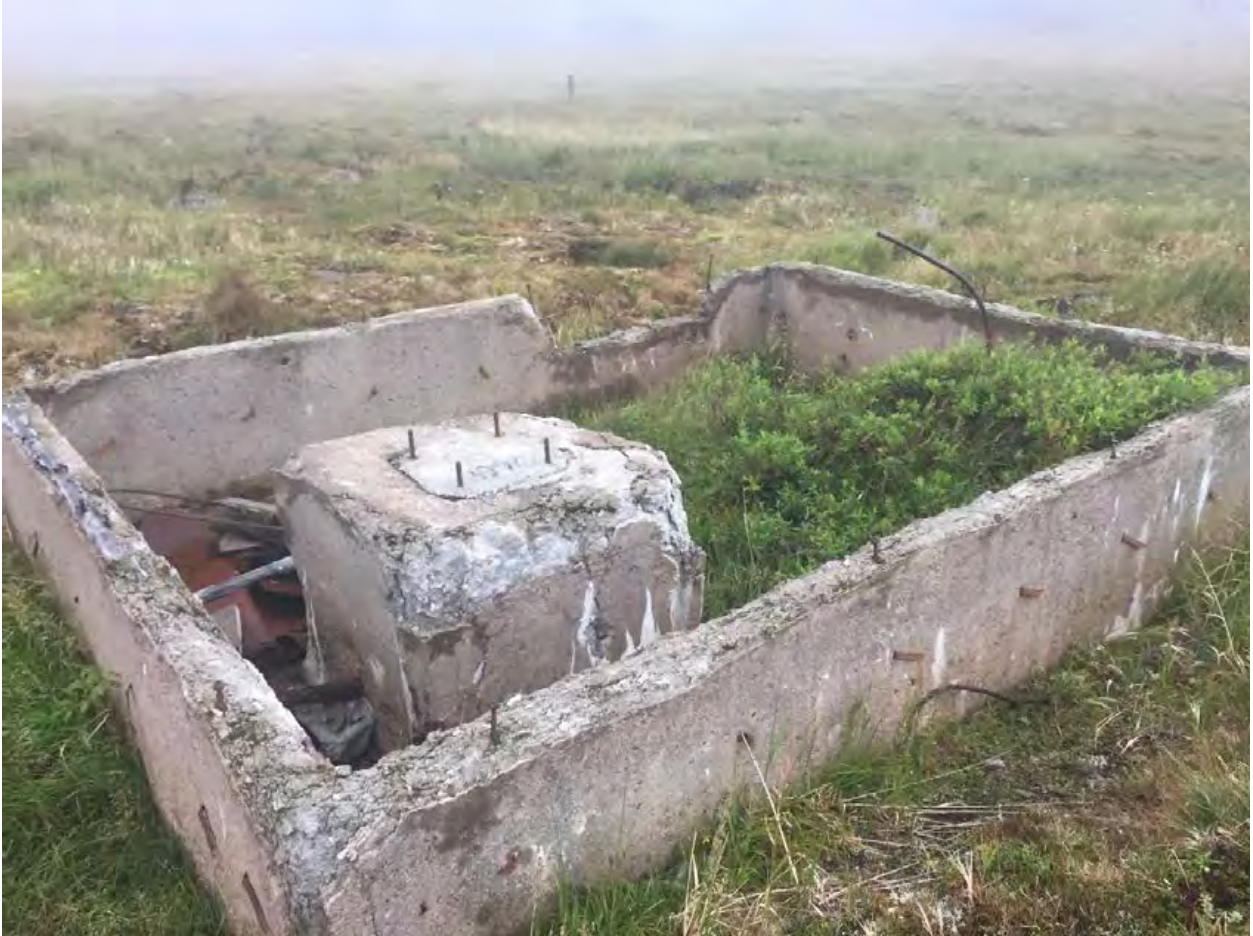
Site SS013 view south west. Concrete foundation in foreground and monitoring well protective casing in background.
