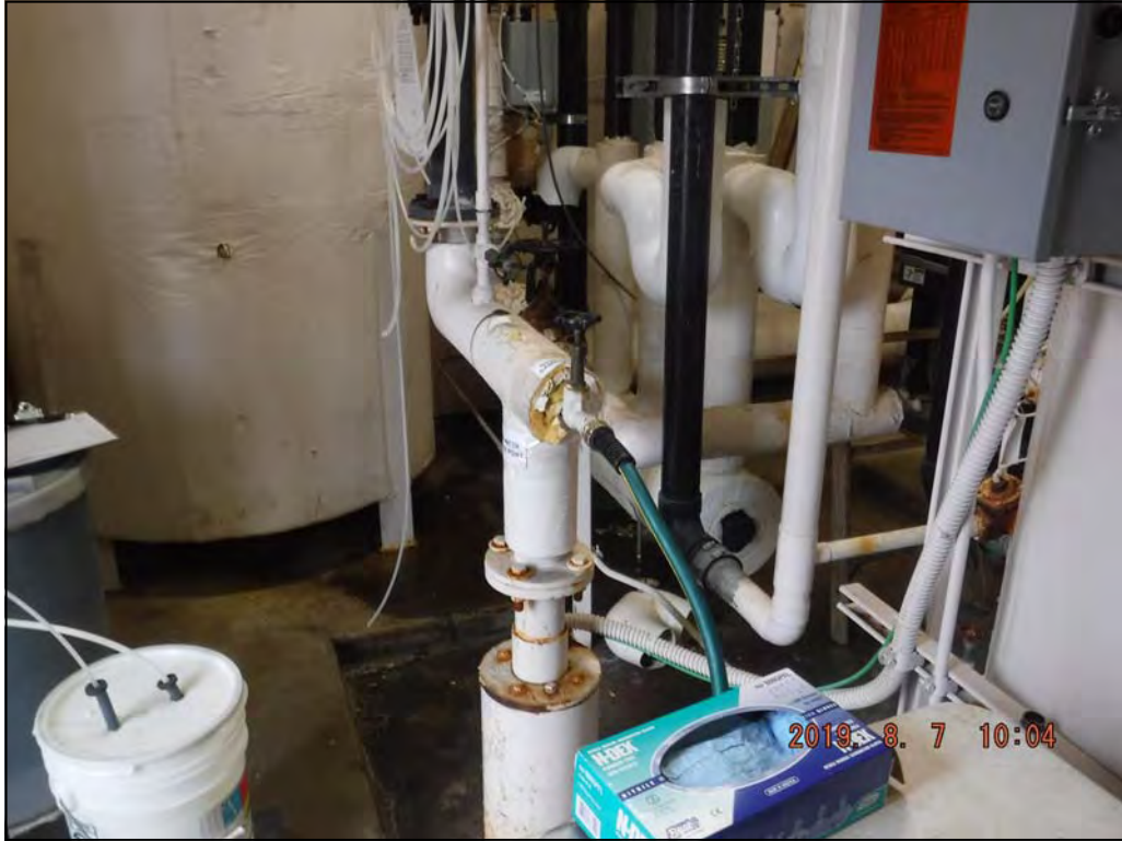
OU2 DRMO — Spigot for the WSW in the Building 5009 Well House (view N/A)
