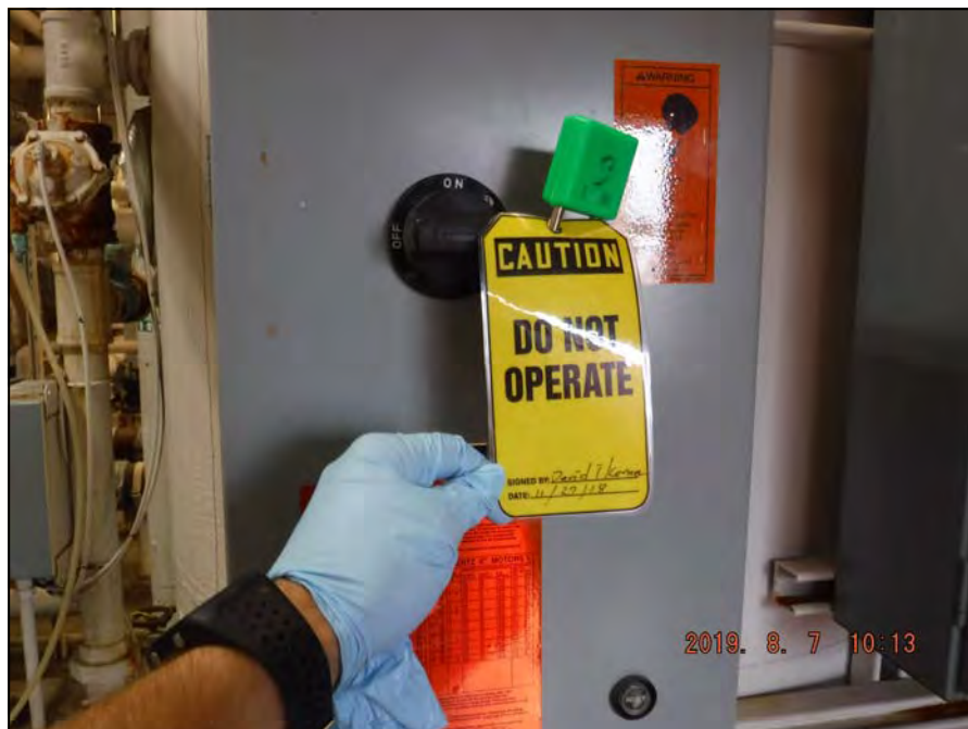
OU2 DRMO — Pump lockout for the Water Supply Well (view N/A)
