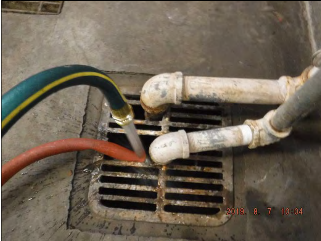
OU2 DRMO — Discharge of purge water into the floor drain at the Building 5009 Well House (view N/A)
