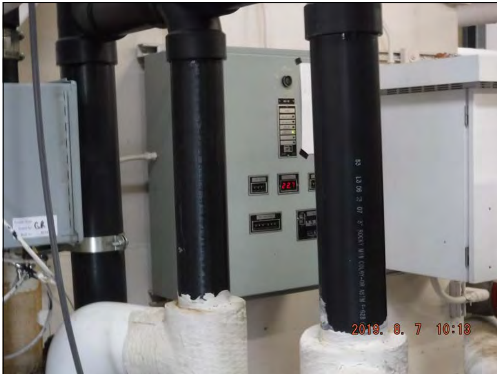
OU2 DRMO — Pump controller for the WSW in the Building 5009 Well House (view N/A)
