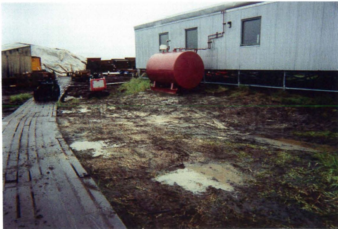
Area C and Area D excavations following backfill activities. Photograph taken by Denise Daggett.
