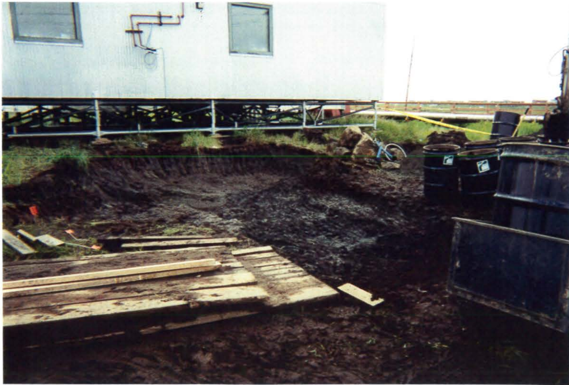
Area C excavation following removal of DRO contaminated soil. Photograph taken by Denise Daggett.
