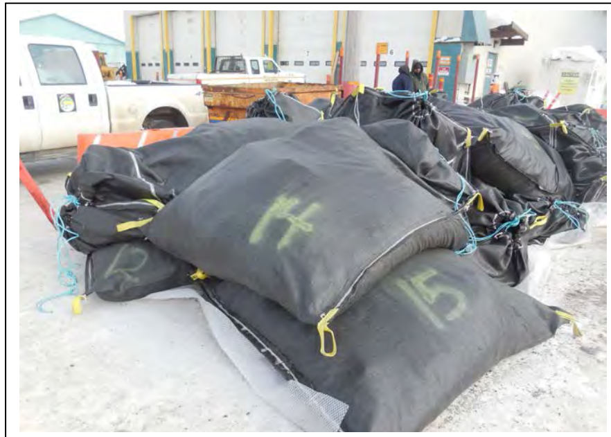
Photo 14: Excavated soils were bagged and placed on a liner at the northeast end of the Shop #2 site; facing southeast. (April 18, 2015)
