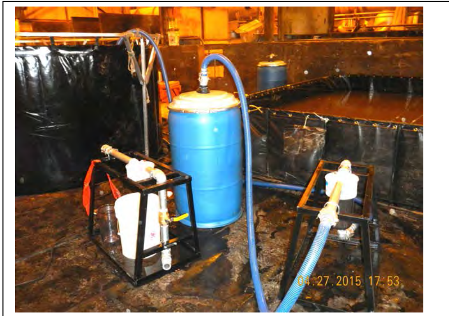
Photo 16: The GAC filtration system setup. Water in the 2,000-gal holding tank is filtered water from the round holding tank (Pictured on the left behind the GAC setup). (April 27, 2015)
