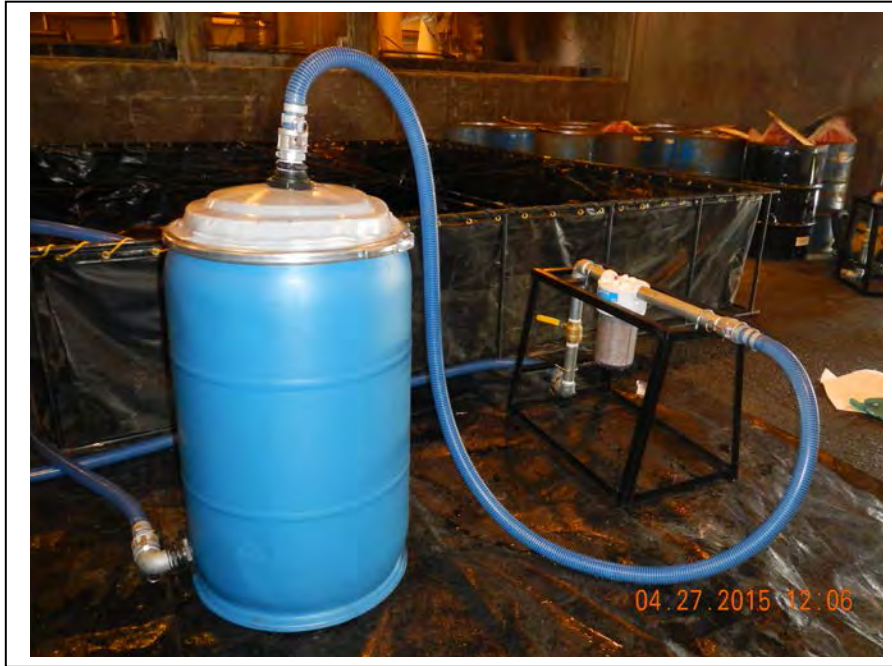
Photo 15: 55-gallon granular activated carbon (GAC) drum (on the left) and micron filter (on the right), in front of the 2,000-gallon holding tank. (April 27, 2015)
