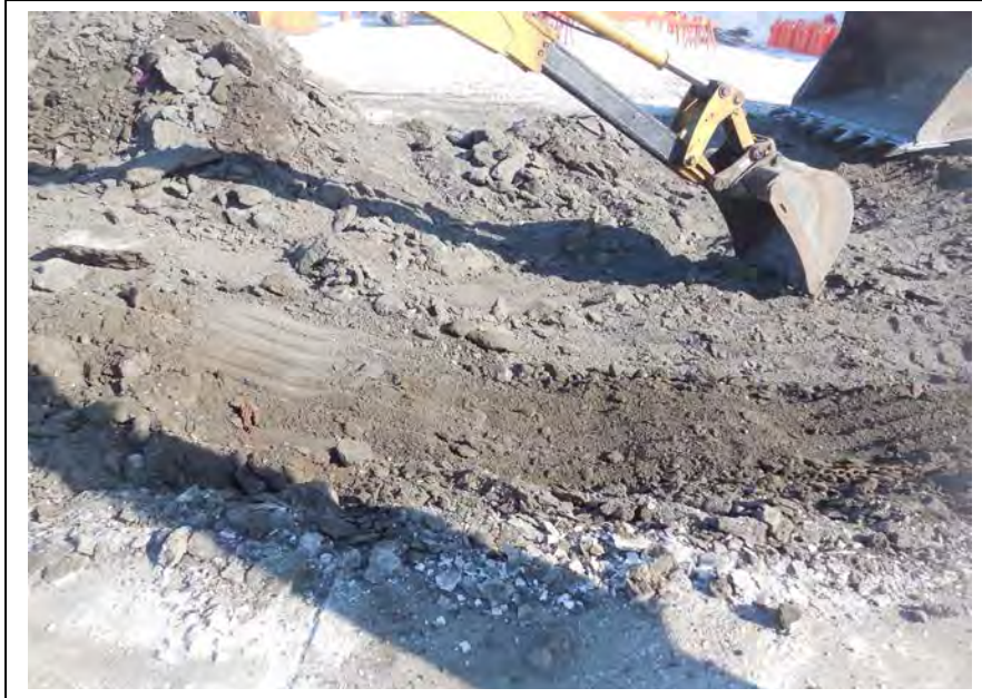
Photo 11: Staining was observed in the west corner of the fuel release area (E1); facing east. (April 17, 2015)
