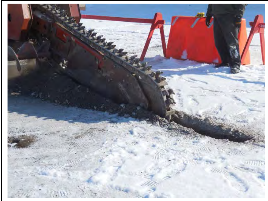
Photo 7: The ULSD fuel release area (E1) was trenched with a trencher in order to break up frozen soil prior to excavation. (April 16, 2015)
