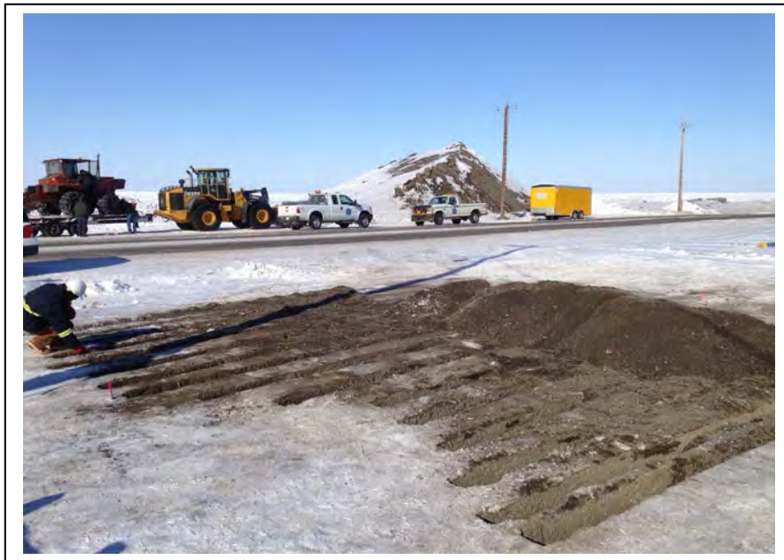
Photo 8: Barrow Utilities trenched soil in the fuel release area (E1) to approximately six to eight inches bgs, separating the trenches by approximately one foot; facing north towards Stevenson Street. (April 16, 2015)
