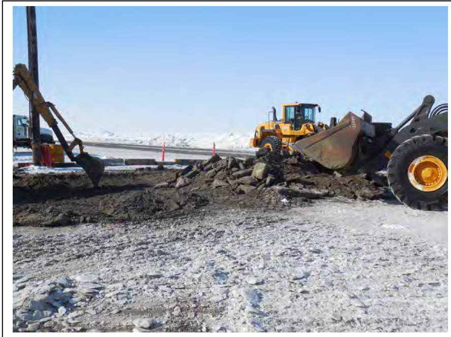
Photo 9: NSB crews used a loader and small backhoe to break up and excavate contaminated soil in the fuel release area (E1); facing west-southwest towards Stevenson Street. (April 17, 2015)
