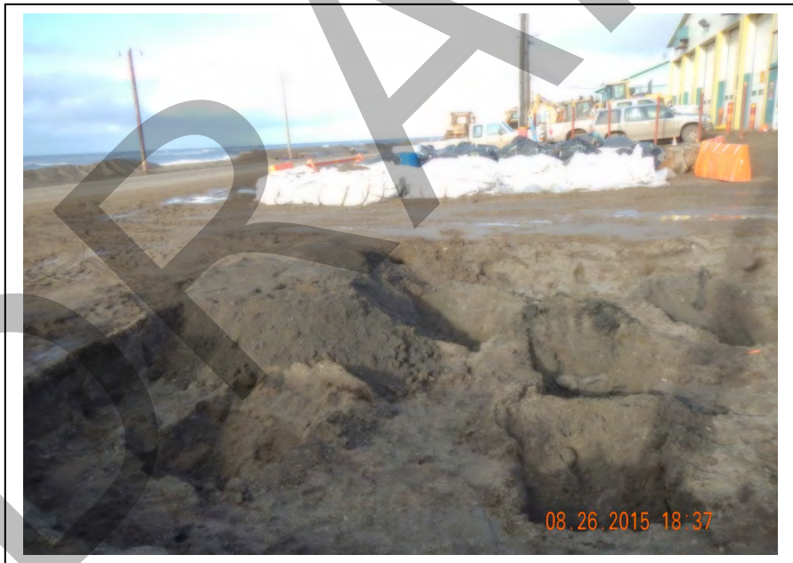
Photo 31: Test pits dug in the base of the excavation to allow for additional field screening (August 26, 2015).
