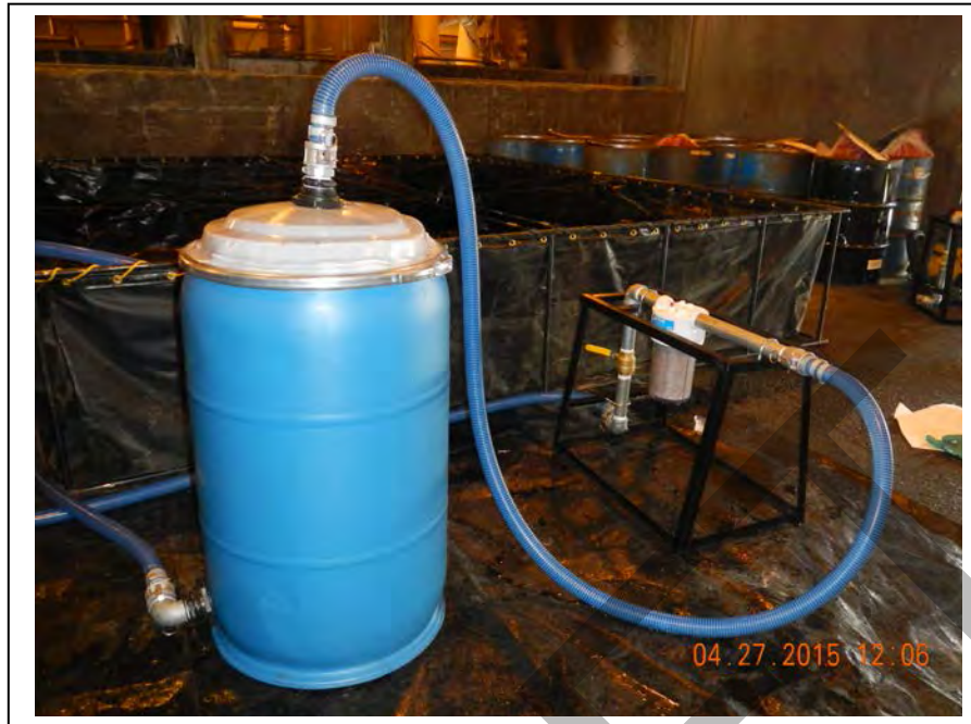
Photo 15: 55-gallon granular activated carbon (GAC) drum (on the left) and micron filter (on the right), in front of a 2,000-gallon holding tank (April 27, 2015).
