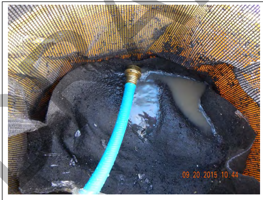
Photo 51: Snowmelt water from the fast tank purging into a scrubber unit setup at NSB Shop #2 (September 20, 2015).
