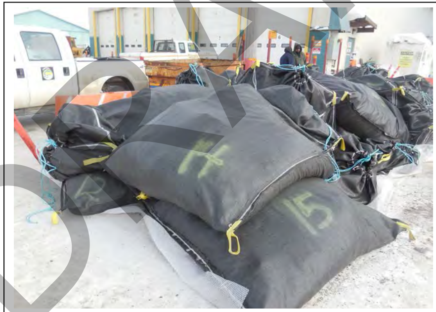
Photo 14: Excavated soils were stored in supersacks and placed on a liner at the northeast end of the Shop #2 site; facing southeast (April 18, 2015).
