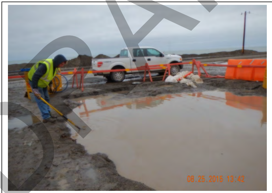
Photo 25: Excavation site flooded after a heavy precipitation event (August 26, 2015).
