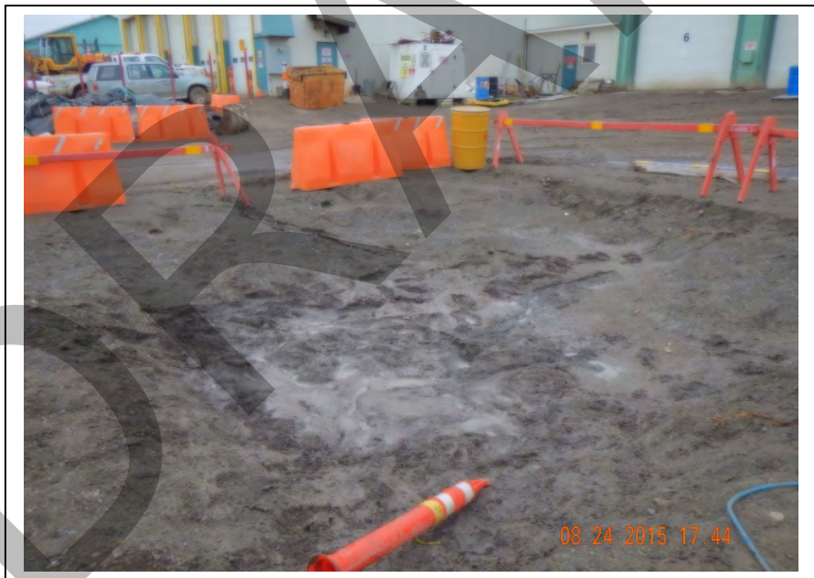
Photo 29: Excavation site after all the standing water was pumped into containment (August 24, 2015).
