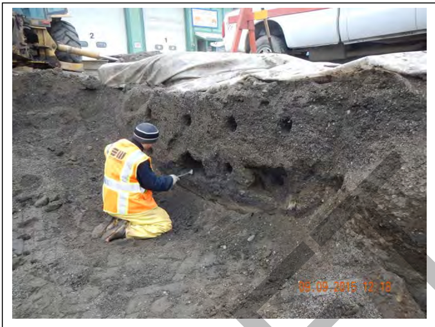
Photo 42: Manual removal of small clay deposits producing substantially higher PID readings than surrounding material; facing southwest (September 9, 2015).
