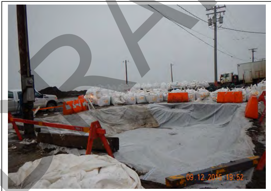
Photo 47: Excavation site secured and supersacks containing excavated soil numbered and tagged; facing north (September 12, 2015).
