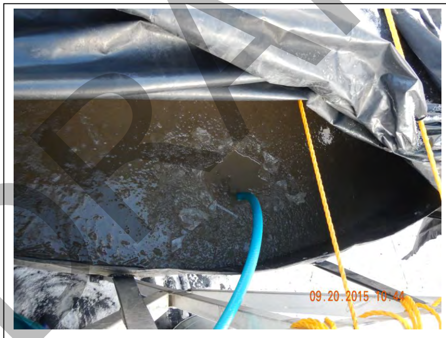
Photo 49: Purge hose setup for gravity discharge of storm water inside the fast tank (September 20, 2015).
