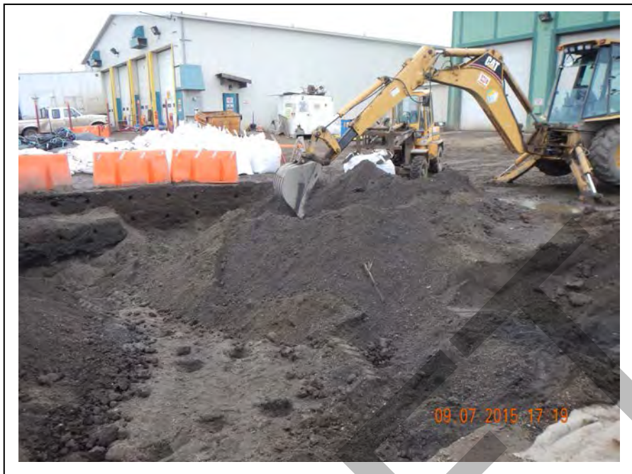
Photo 36: Excavation expanded after field screen results showed additional petroleum contamination; facing south east (September 7, 2015).
