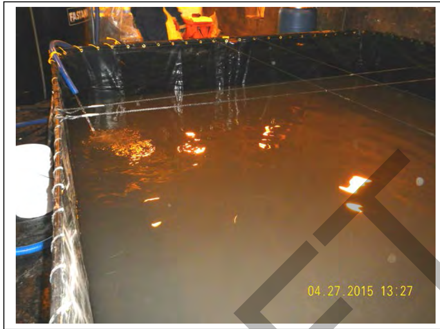
Photo 19: Effluent water from the GAC filtration system stored in a 2,000 gallon holding tank (April 27, 2015).
