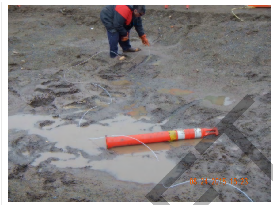
Photo 28: NSB personnel using a peristaltic pump to drain shallow puddles of potentially contaminated water (August 24, 2015).
