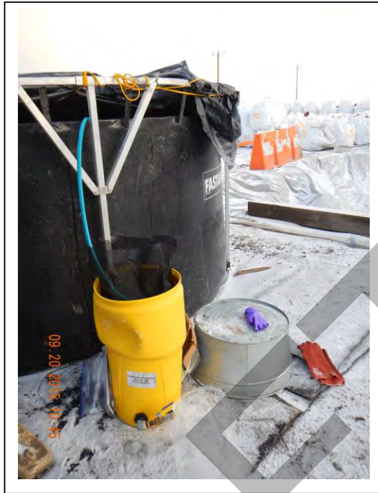
Photo 50: GAC unit setup for treatment of snowmelt water inside the covered fast tank at Shop #2 (September 20, 2015).
