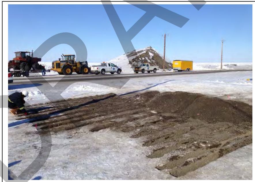
Photo 8: NSB trenched the soil in the fuel release area (E1) approximately six to eight inches below ground surface (bgs), separating the trenches by approximately one foot; facing north towards Stevenson Street (April 16, 2015).
