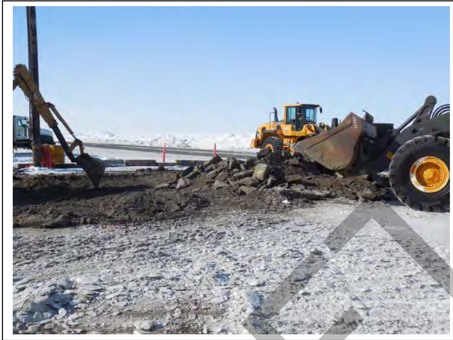
Photo 9: NSB crews used a loader and backhoe to excavate potentially-contaminated soil in the fuel release area (E1); facing west-southwest towards Stevenson Rd (April 17, 2015).
