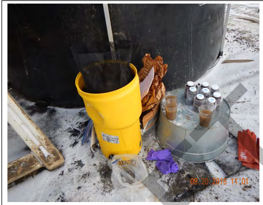
Photo 52: Scrubber unit setup for treatment of snowmelt water inside the covered fast tank at Shop #2 (September 20, 2015).
