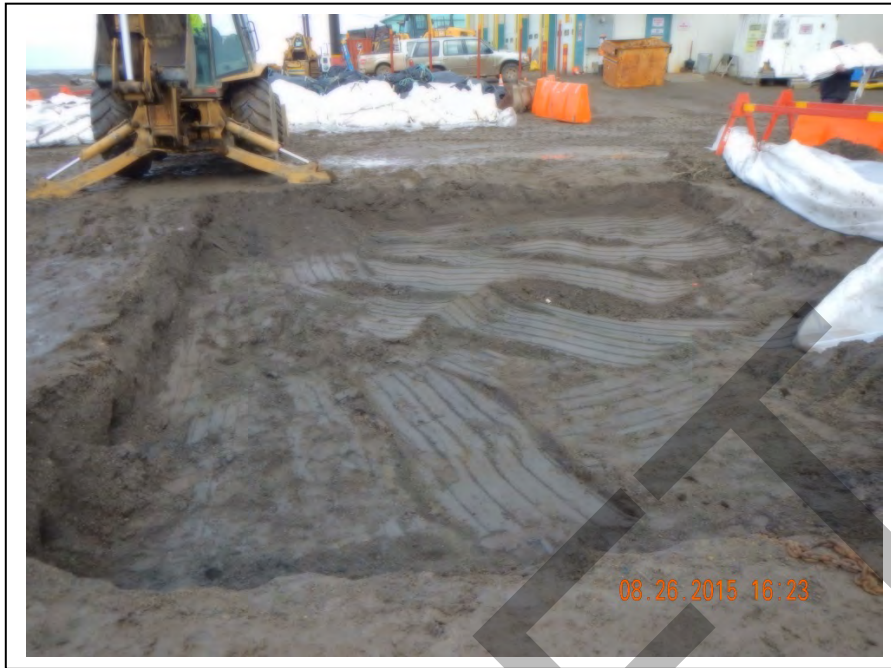
Photo 30: Excavation site with approximately the first foot of potentially-contaminated soil removed (August 26, 2015).
