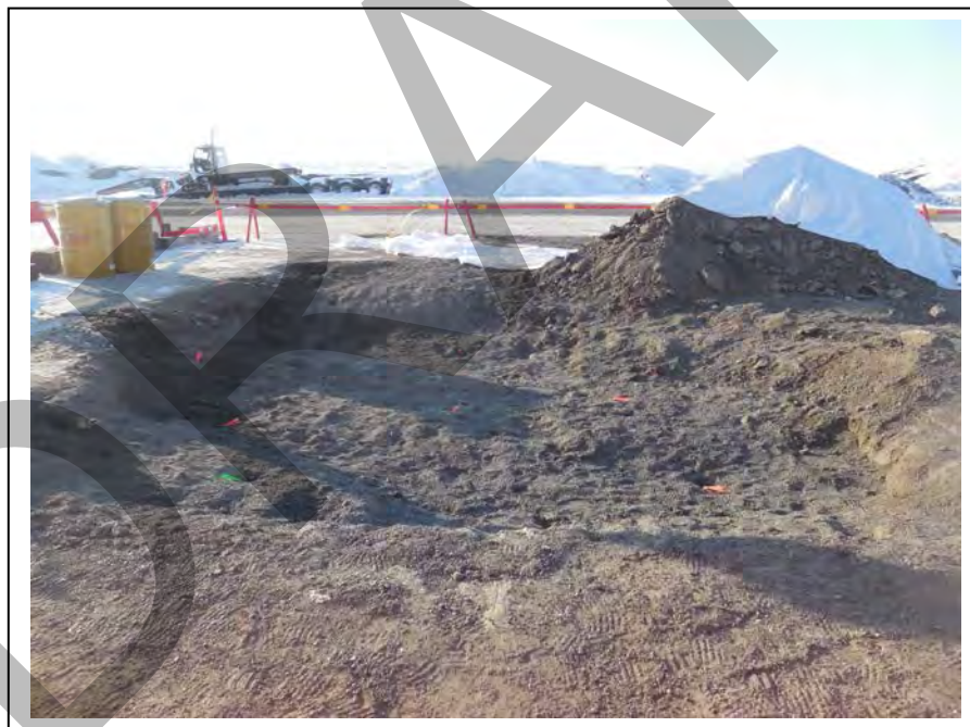
Photo 12: Analytical soil samples were collected from the base and sidewalls of the excavated area; facing northwest towards Stevenson Rd (April 18, 2015).
