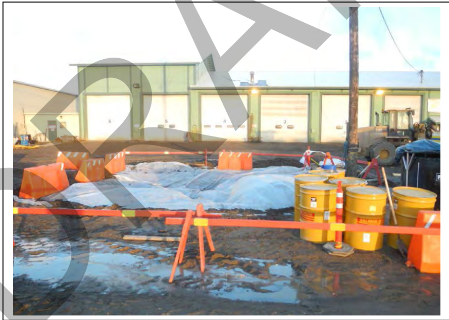
Photo 33: Excavation site covered by a liner to prevent additional quantities of runoff water from coming into contact with potentially-contaminated soil (August 26, 2015).
