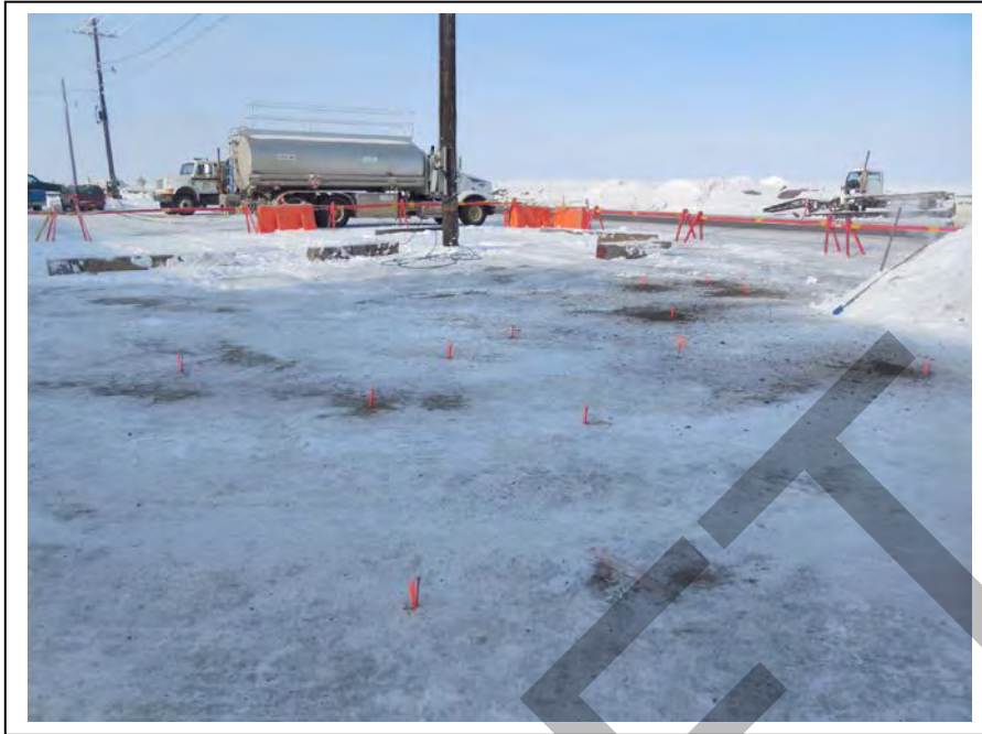
Photo 5: Site characterized with 14 field-screen-locations in the fuel release (E1) area and six locations in the snow stockpile area (E2); locations marked with survey markers (April 15, 2015).
