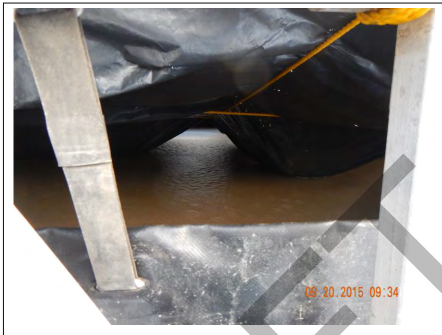
Photo 48: Ice layer, approximately two – five inches thick inside covered fast tank at Shop #2 (September 20, 2015).
