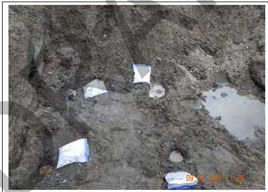
Photo 41: Water was observed seeping into the field screening locations within several minutes of being dug (September 6, 2015).
