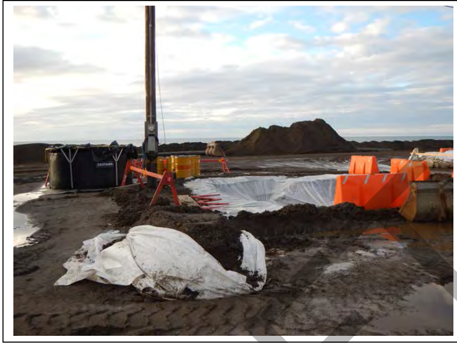
Photo 34: Project site at the start of additional excavation activities; facing north by northwest (September 2, 2015).
