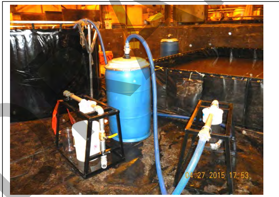
Photo 16: The GAC filtration system assembled. Untreated water in the FASTANK on the left is filtered through the GAC system into the 2000 gallon holding tank on the right (April 27, 2015).
