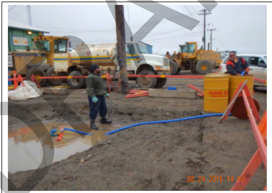
Photo 27: Pumping approximately 200 gallons of potentially contaminated water into three 85-gallon drums (August 24, 2015).
