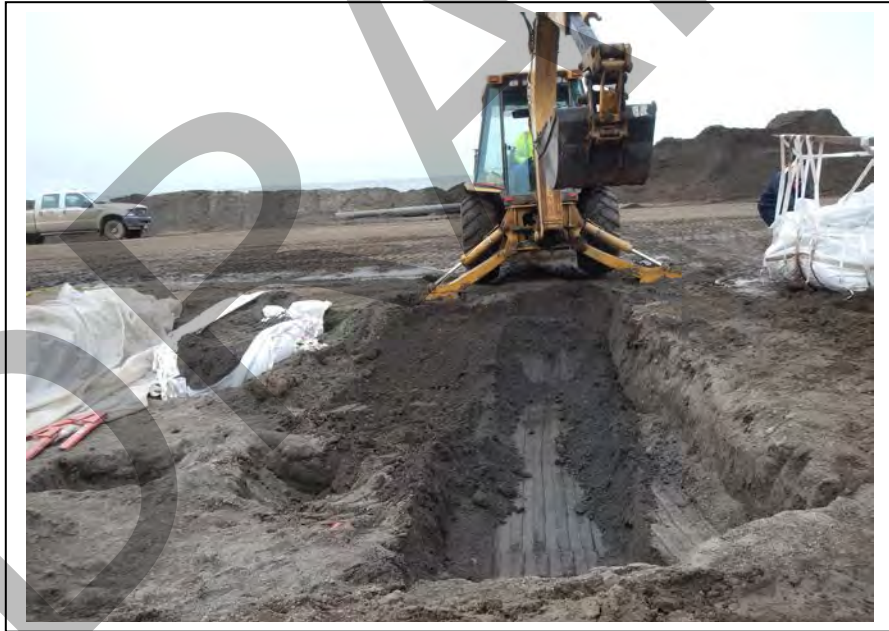
Photo 35: Intermittent staining observed in the soil profile; facing northwest (September 4, 2015).
