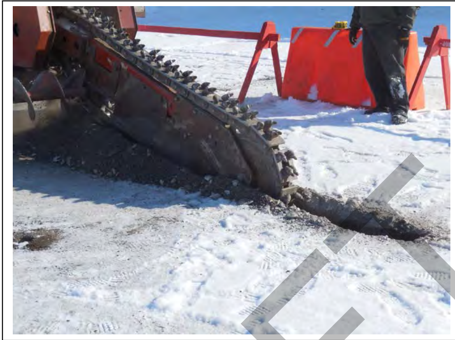
Photo 7: The ULSD fuel release area (E1) was trenched with a rock saw in order to break up frozen soil prior to excavation (April 16, 2015).
