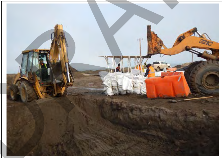
Photo 39: Excavated soil were placed in 2 and 5-cubic yard supersacks; facing north (September 5, 2015).
