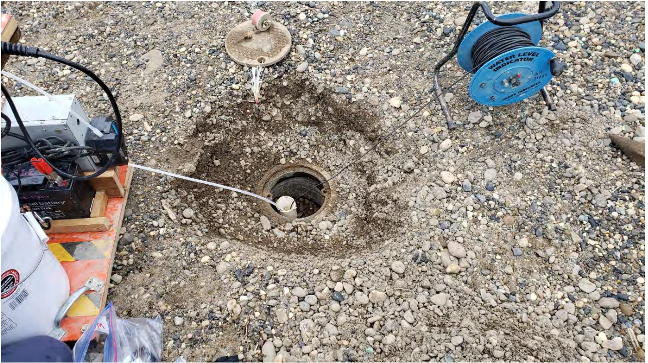
Photo 4: Monitoring Well MW-4R: The frost-jacked two-inch PVC well casing was cut down following sample collection.
