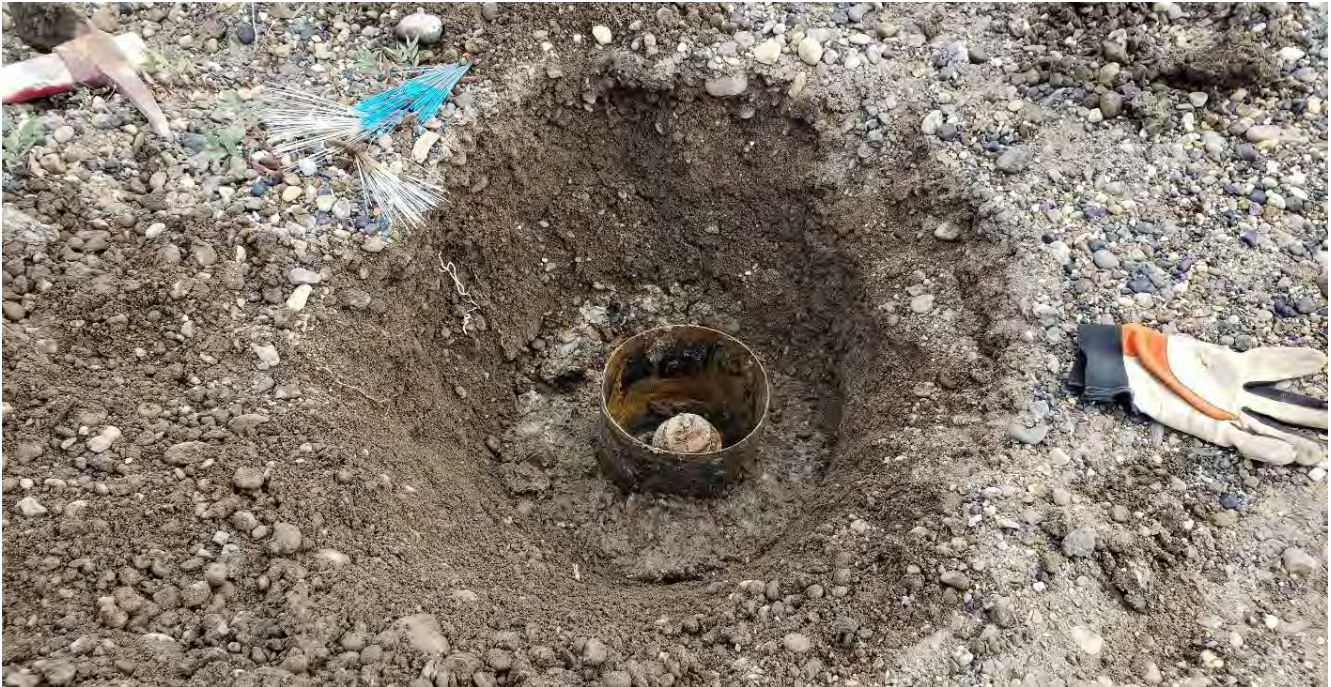
Monitoring well MW-22: The monument was raised to approximately ten inches below the ground surface (bgs). Bentonite was added in the area surrounding the monument. The bentonite was hydrated to prevent surface water from infiltrating the well monument. (July 18, 2019).
