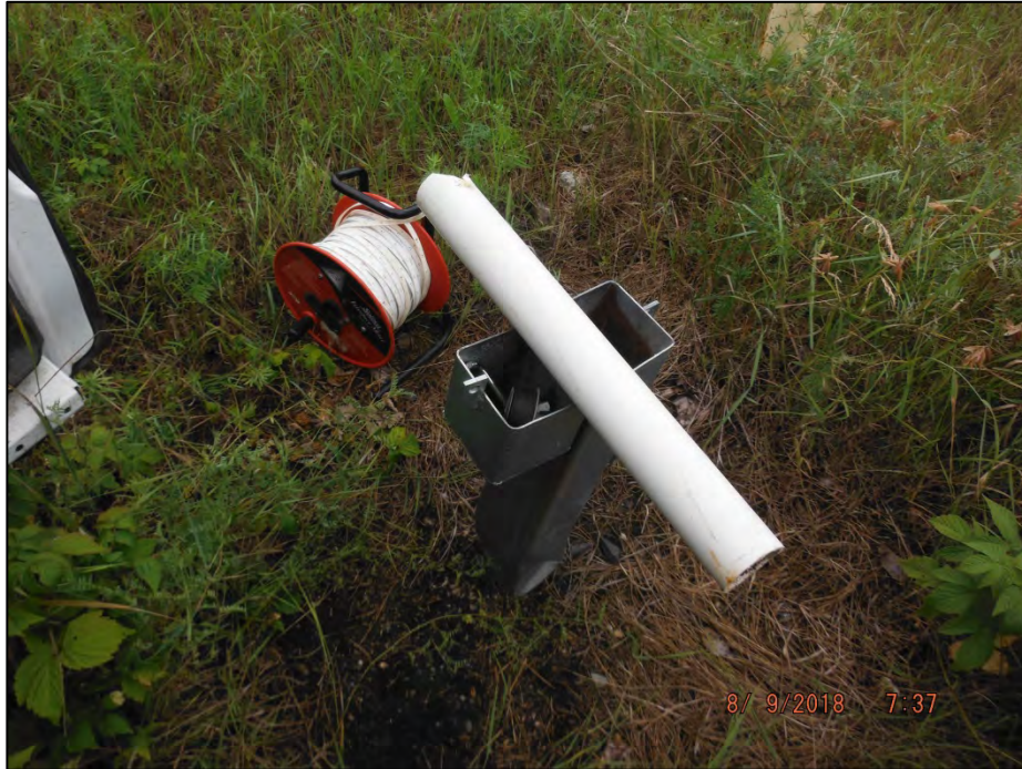
Broken casing at Monitoring Well AP-7187
