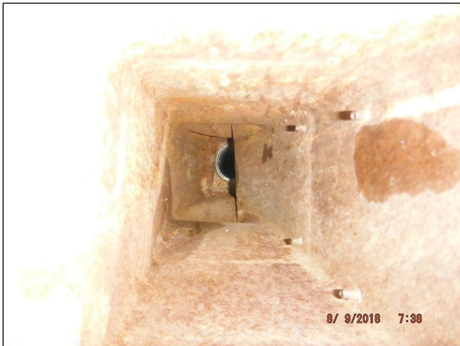
View inside Overcasing of Monitoring Well AP-7187
