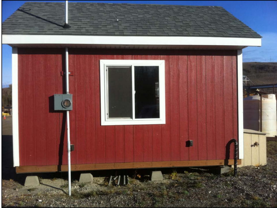
PHOTOGRAPH 3: VIEW OF THE “WELL HOUSE” AND OUTSIDE SPIGOT (RIGHT SIDE OF PHOTO), LOOKING NORTH (SEPT 2011)
