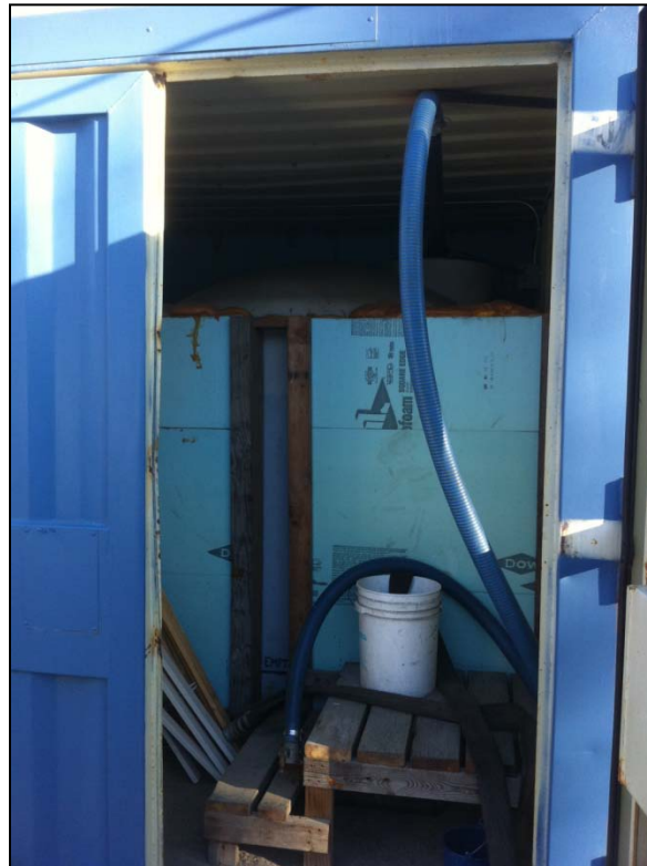
PHOTOGRAPH 2: VIEW INSIDE WATER BIN STORAGE CONNEX (SEPT 2011)
