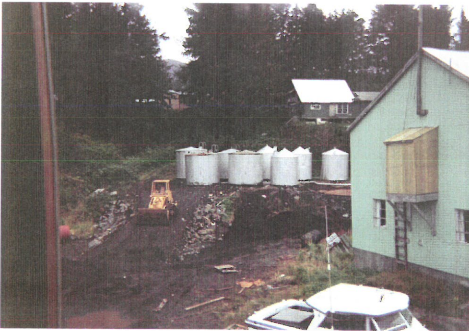
Port Graham tank farm, viewed from window of general store.
