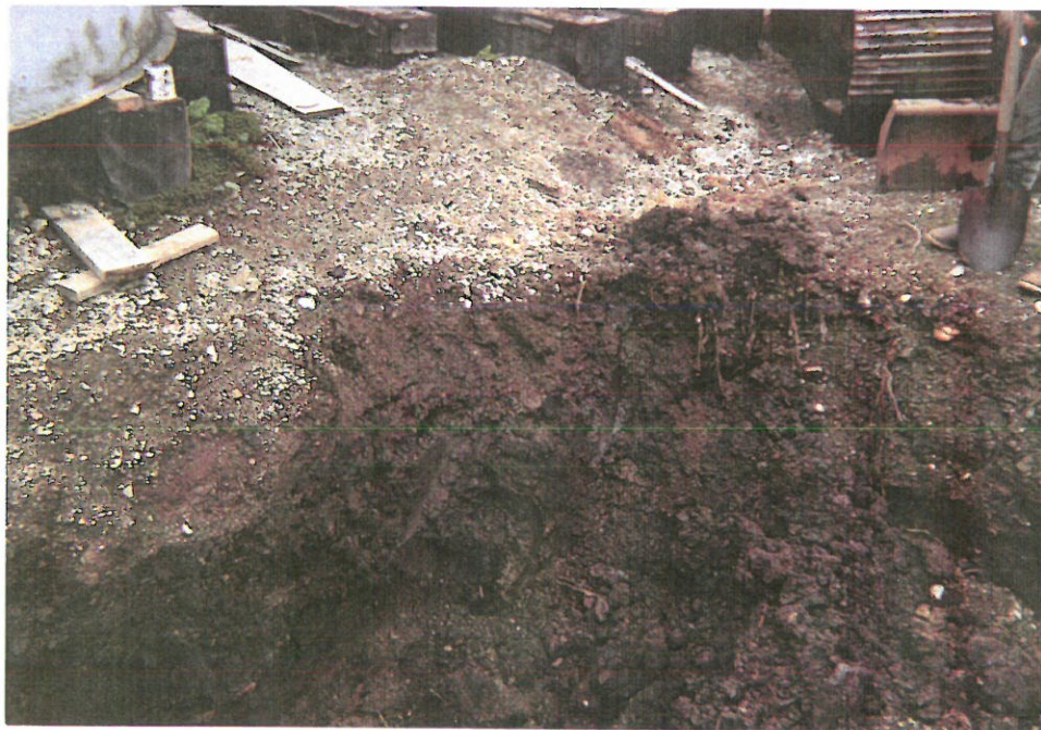
Seep exposed during excavation of test pit number six
