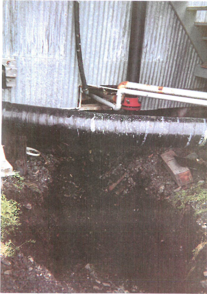
Test pit number one, western wall of cannery building, directly beneath product piping, adjacent to excavation "A". This was apparently the location of an abandoned septic tank leach field.
