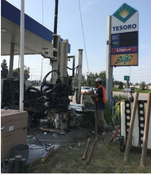
Photo 1: Drilling RM-2 Well with Geoprobe 8040DT track mounted drilling rig operated by GeoTek Alaska, July 2019
