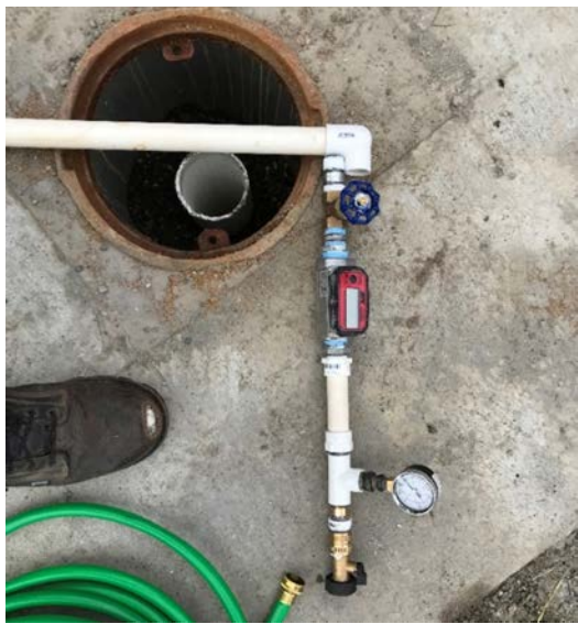
Photo 3: Top view of completed 4" diameter PVC well casing inside 12" diameter steel flush mounted protective casing in concrete slab and piping for well pump testing, August 2019
