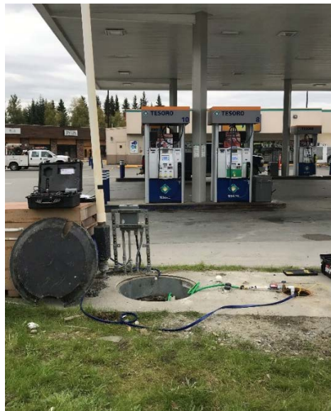
Photo 4: Looking south at fuel dispenser islands during well development of RM-2 (in foreground) with discharge hose to Chemox injection wells inside manhole to the right of knock box, August 2019
