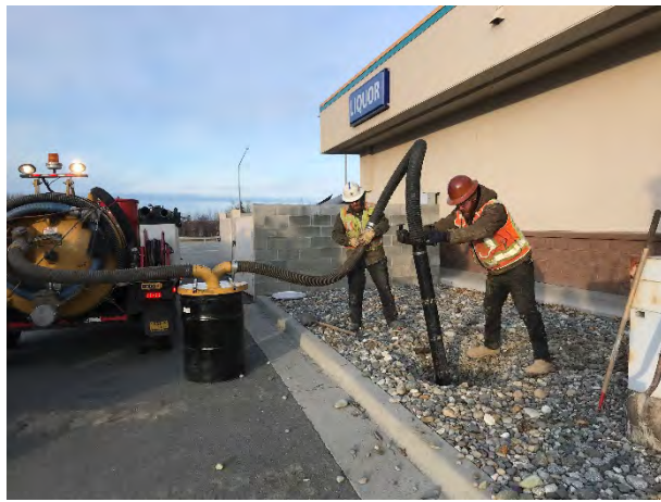
Photo 1: Vacuuming the upper 5-feet of soil prior to start of drilling RW 19-1 well
