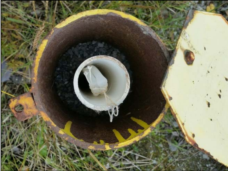
Tubing, which was removed and disposed of, found within MWA22.
