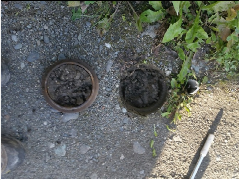
DPB21 broken PVC casing partially filled with dirt.
