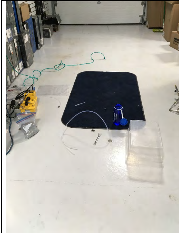
Curing of sub-slab monitoring point, and monitoring point for cross-slab pressure differentials in the background
