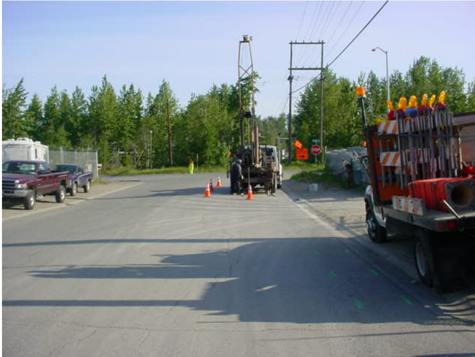
Photograph 1: Looking north on North Sitka Street, Boring B1 was advanced as close to Viking Drive as utility locates allowed. Photo taken on June 14, 2007.
