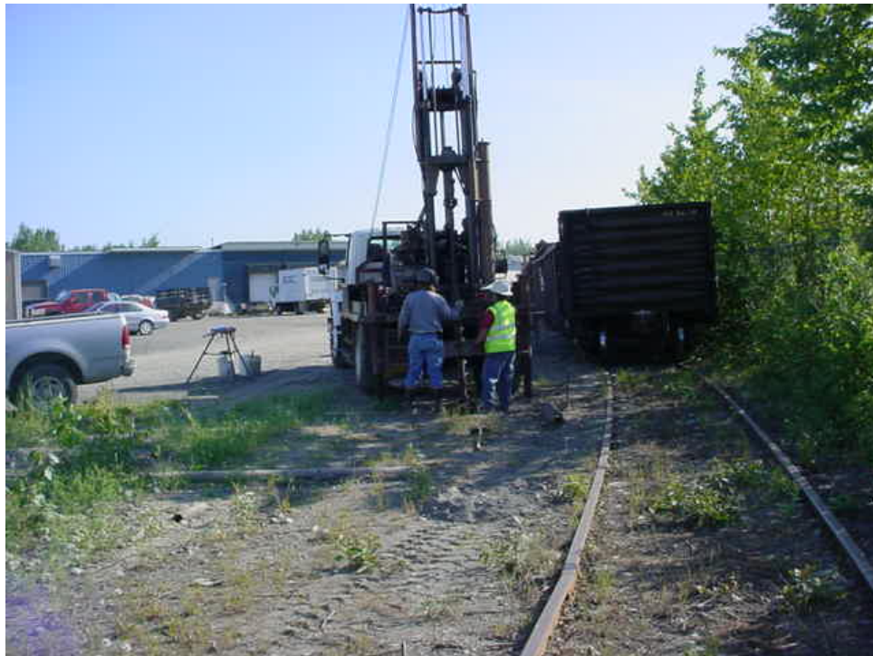
Photograph 5: Looking northeast. Advancing Boring B11 along railroad ROW. Photo taken on June 14, 2007.
