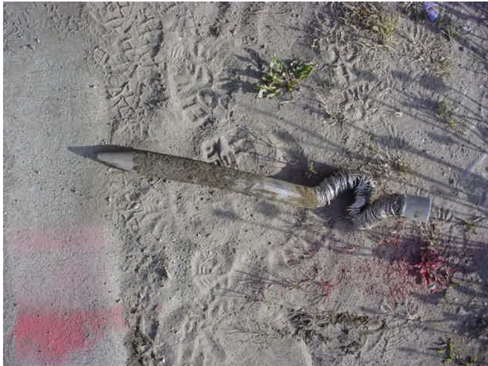
Photograph 2: Damaged wellpoint from attempt at driving into Boring 2. Photo taken on June 14, 2007.
